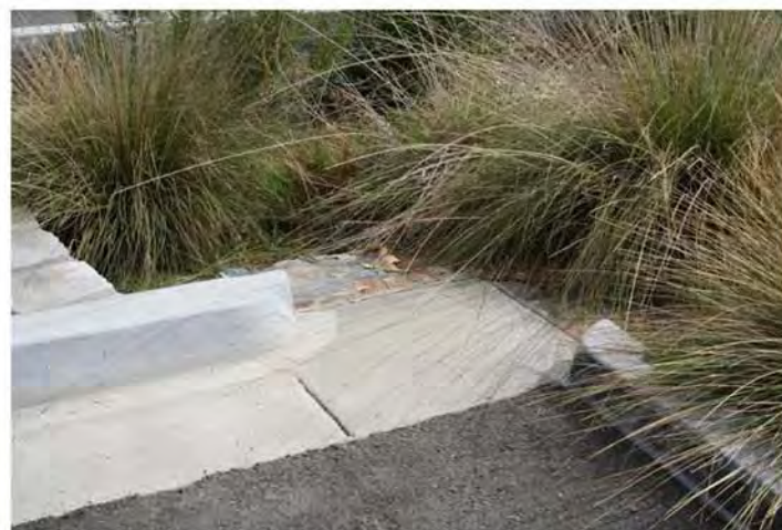
GAP IN CURB DIRECTS STORMWATER TO PLANTS
