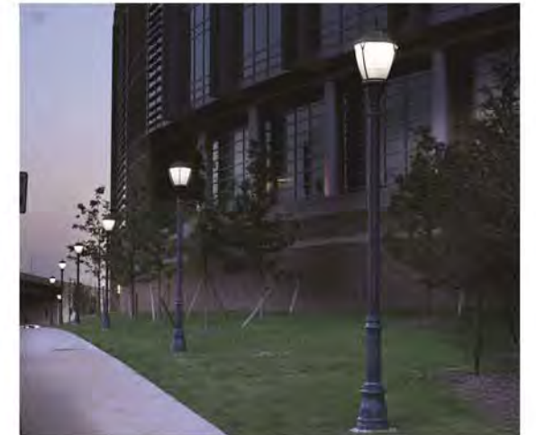
PEDESTRIAN SITE LIGHTING
