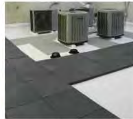
ROOF WALKWAY AND CONDENSER UNITS
