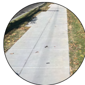
DDOT STANDARD SCORED CONCRETE SIDEWALK
