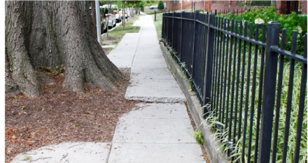
D | Tree roots lift sidewalk panels along 24th Street north of Wagner Street SE
