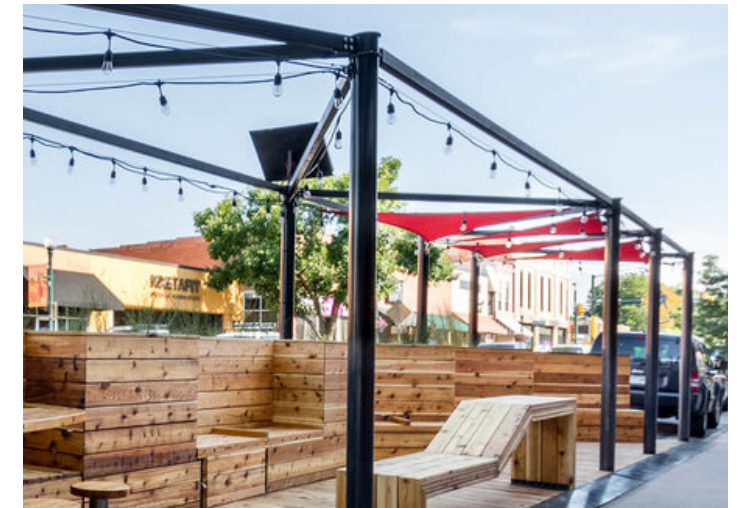
Catenary Lighting on Overhead Structure
