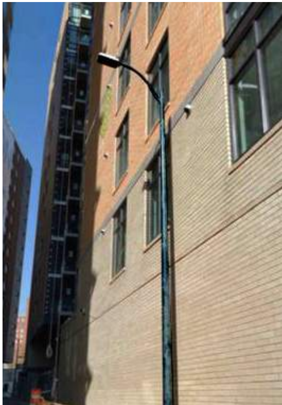
STREET LIGHT: COBRA HEAD - PHILIPS/VALMONT - ROADVIEW LED
