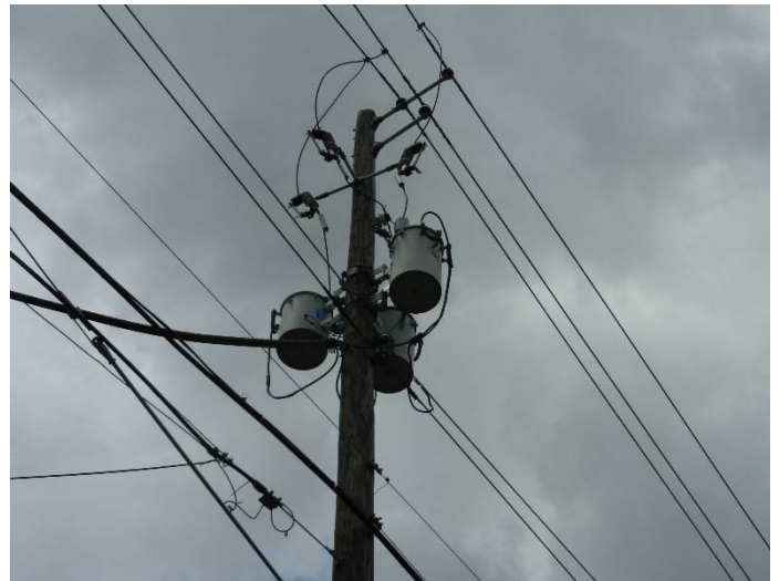
14. View of three adjacent transformers located along Benning Road
