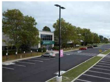
PARKING LOT LIGHTING
