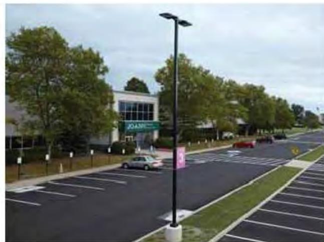
PARKING LOT LIGHTING
