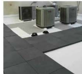
ROOF WALKWAY AND CONDENSER UNITS
