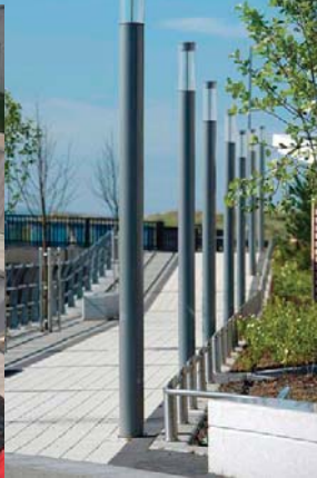
park lighting fixtures
