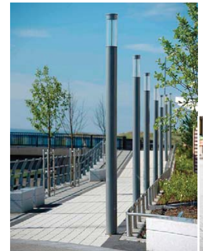
park lighting fixtures
