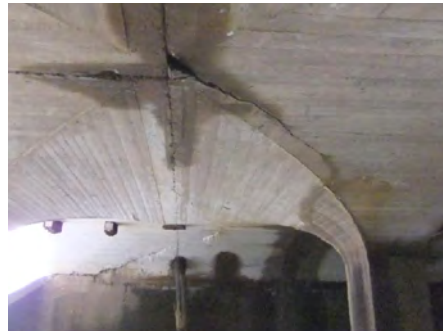
FIG. B.5 -SHIFTING AT THE COLD JOINT AND CONCRETE SPALLING.
