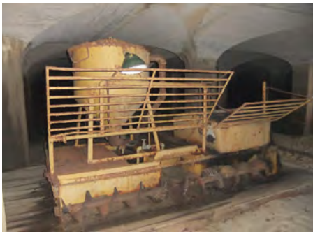
FIG. B.4 - SAND COLLECTING CLEANING EQUIPMENT AT FILTER No. 7.
