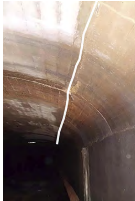
FIG. C.8 - TYPICAL CRACK AT THE BARREL VAULT CEILING NEAR A FILTER END WALL.
