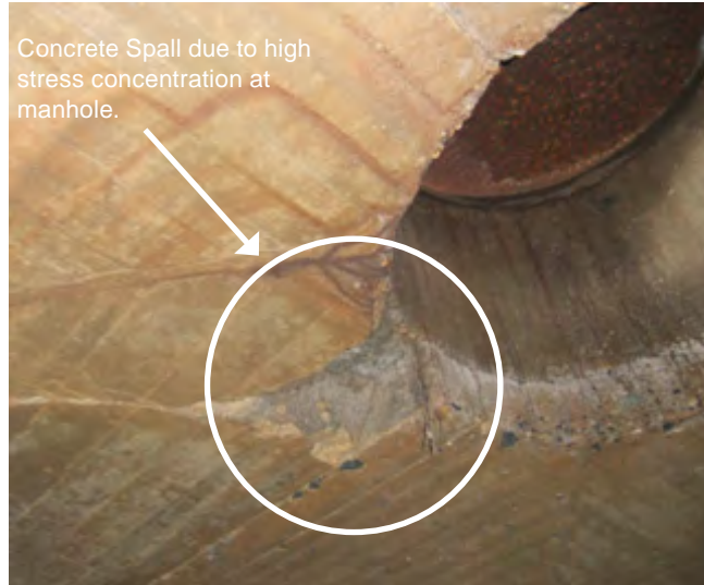
FIG. C.7 - SPALL AT UNDERSIDE OF VAULTED CEILING NEAR MANHOLE.
