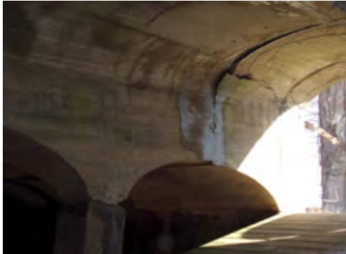
FIG. C.9 - TYPICAL DAMAGE AT ENTRANCE PORTAL.
