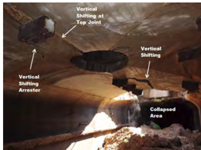
FIG. C.4 - CEILING VAULT DAMAGE NEAR COLLAPSED BAY.
