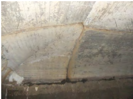
FIG. B.6 - SHIFTING AT VAULTED CEILING JOINT.
