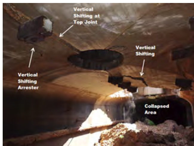
FIGURE 15: CEILING VAULT DAMAGE NEAR COLLAPSED BAY
