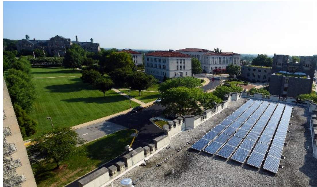
Solar panels on roof of Gibbons Hall
