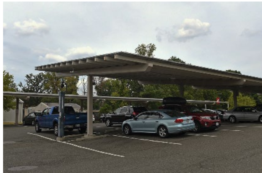
Solar canopy at O'Boyle Parking Lot
