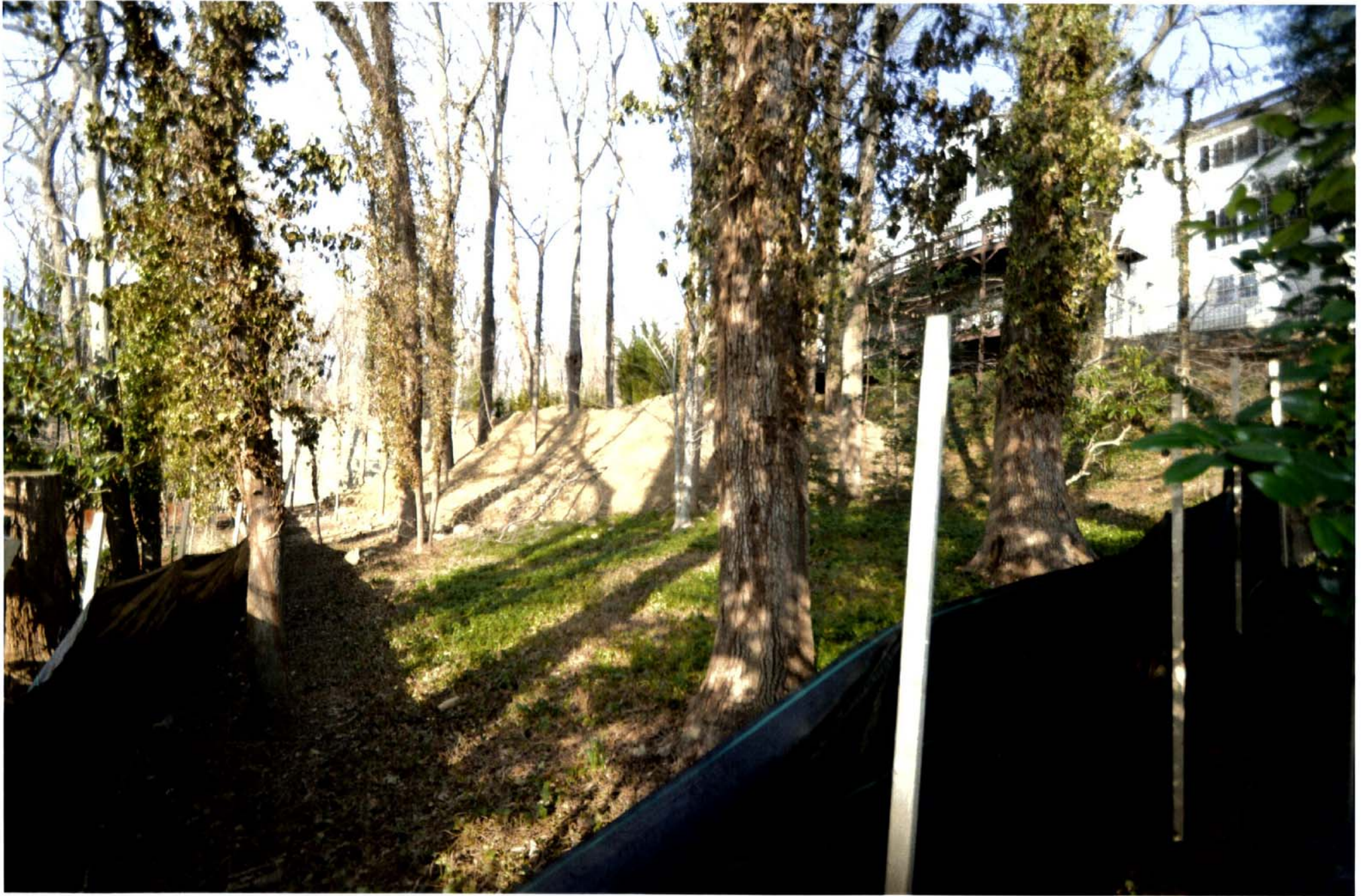
4833 Dexter Terrace, NW, showing no sediment or run-off control at beginning of dumping. March 28, 2014. It still looks much the same, but with more dirt.
