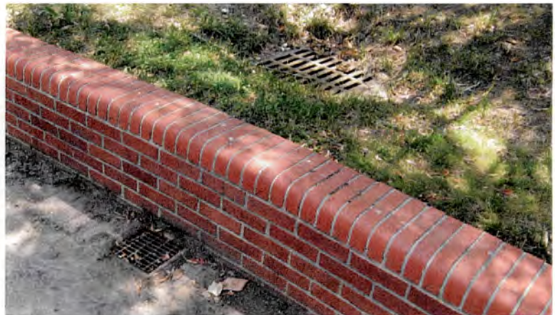
Figure 9 Area drain surrounded by dirt and debris
