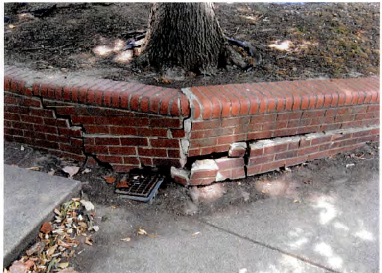
Figure 2 Damaged brick retaining wall
