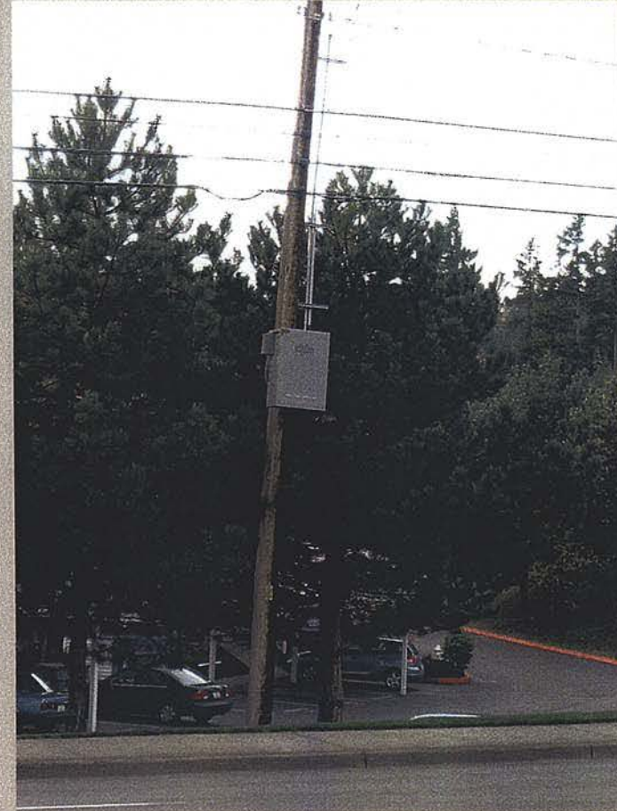
Utility pole in Kirkland
