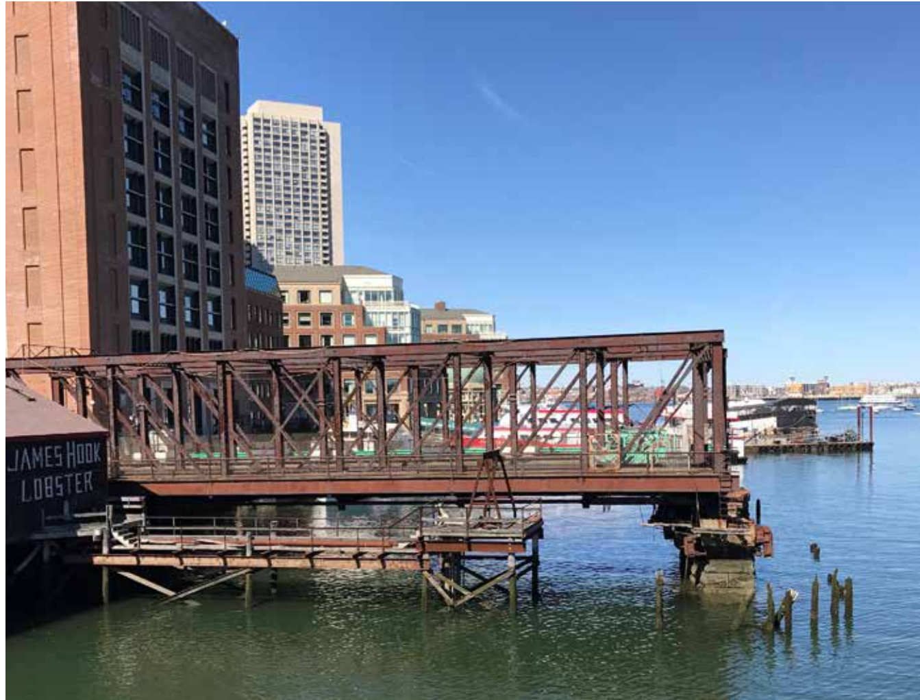
Northern Ave. Bridge, Boston: Expressed structure and materials are hallmarks of maritime construction.
