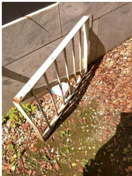
Fig. 108. Metal gate to the utility area at the north façade of the Embassy. The gate does not have a latch, and it does not prevent access to the utility area (LE075).
