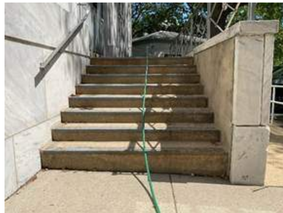
Fig. 86. View north toward the MCAC. Marble veneer on the stair wall is in disrepair, and the stairs do not meet accessibility standards (LE053).
