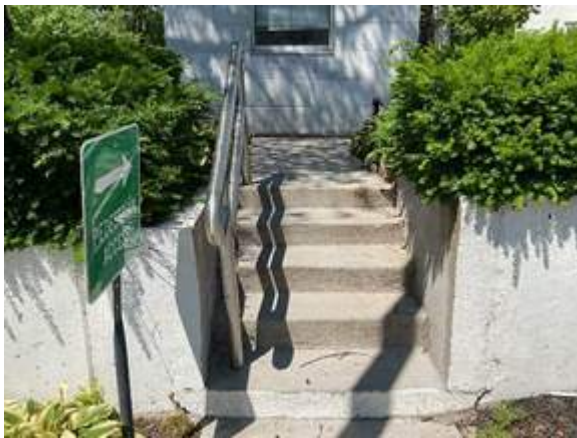
Fig. 53. Pedestrian access stairway to the BCAC guard house does not meet ADA standards (LE041).
