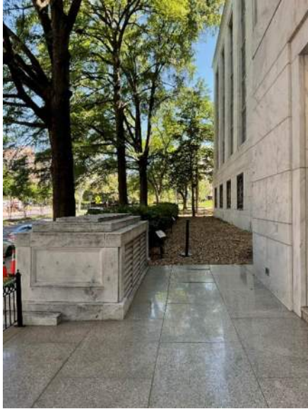
Fig. 9. View north from WCAC entrance upper stairway landing toward loose aggregate strip at foundation (LE011)
