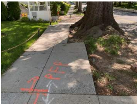
Fig. 29. View east along F Street N.W. The sidewalk buckles at the largest tree on site, a 3.8 m (151 inches) circumference willow oak ( Quercus phellos ), root flare capture at the bottom right corner (LE018).
