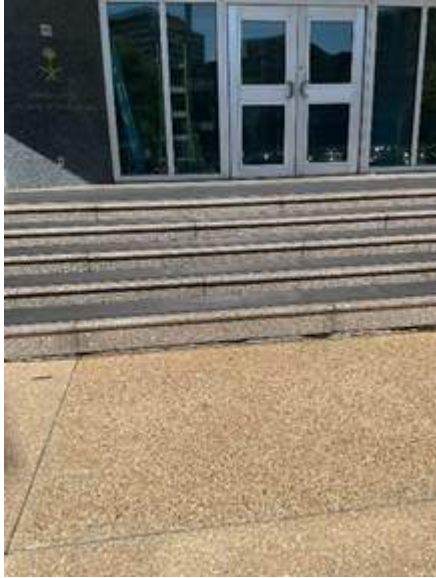
Fig. 77. A wide gap between the stone stairs and exposed aggregate paving reveals settlement of the paving and deteriorating joint material (LE045).
