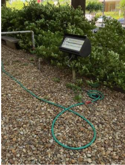
Fig. 13. Hose bib connection and uplight in loose aggregate strip south of WCAC entrance (LE011)
