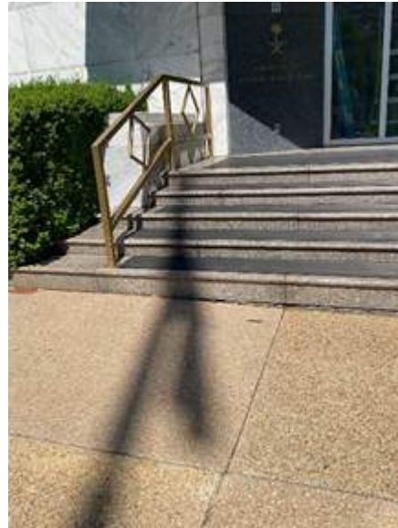
Fig. 76. Exposed aggregate paving and stone stairs to the main entrance at the southeast façade. Rubber mats for slip resistance are warping and creating a trip hazard. Stair railing does not meet accessibility standards (LE045).
