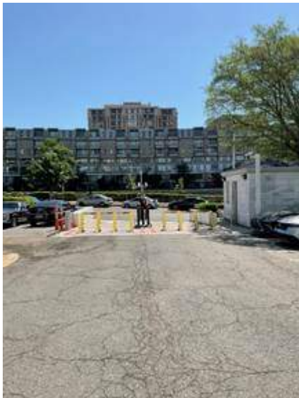
Fig. 67. View east from the parking lot toward the BCAC vehicular screening area and guard house (at right). Cracks spread throughout the asphalt paving (LE055).
