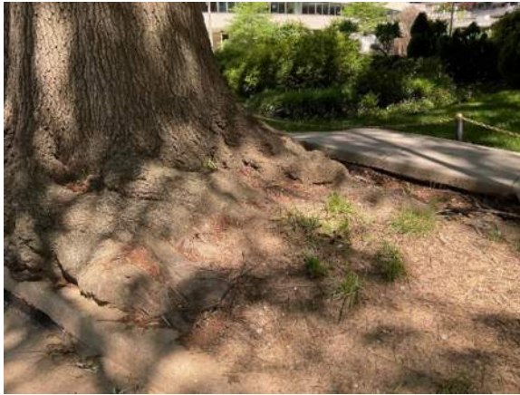
Fig. 31. View northwest along F Street N.W. at the 3.8 m (151 inch) circumference willow oak. The root flare lifts the adjacent concrete sidewalk (LE018).
