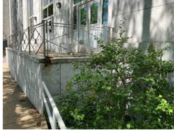
Fig. 88. Small holly at the foundation of the marble stair wall, north of the double doorways on the southeast façade (LE053).
