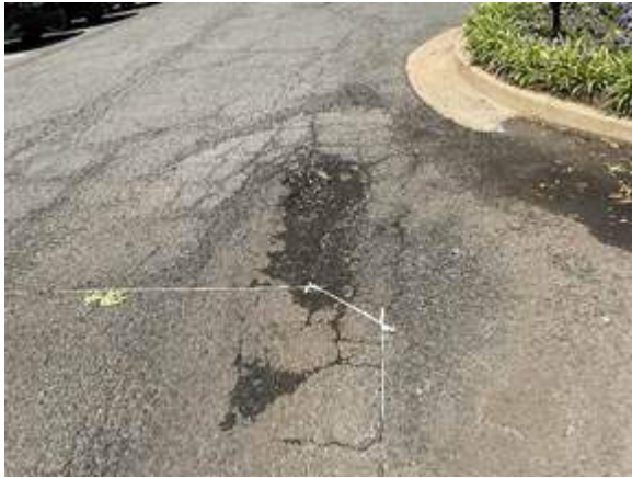
Fig. 65. Cracked asphalt pavement near the flagpole in front of the southeast façade (LE043).
