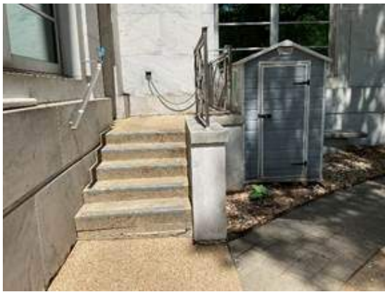
Fig. 83. Stairs lead to a door at the north side of this façade (LE048). A hose bib is located at the top landing. Aggregate paving is cracked and separating from the stair risers. Handrail does not meet accessibility standards. A concrete paver path meets the aggregate paving at right (LE049). A small shed sits in a bed of loose aggregate (LE050).
