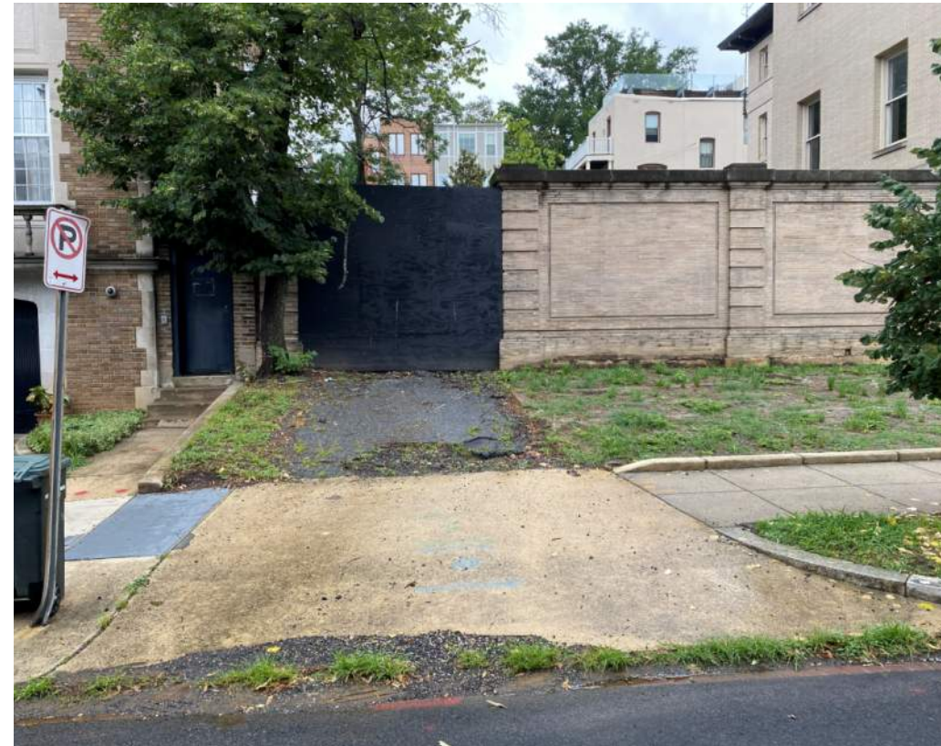
EXISTING DRIVEWAY FROM R STREET, NW & WALL CONDITION
