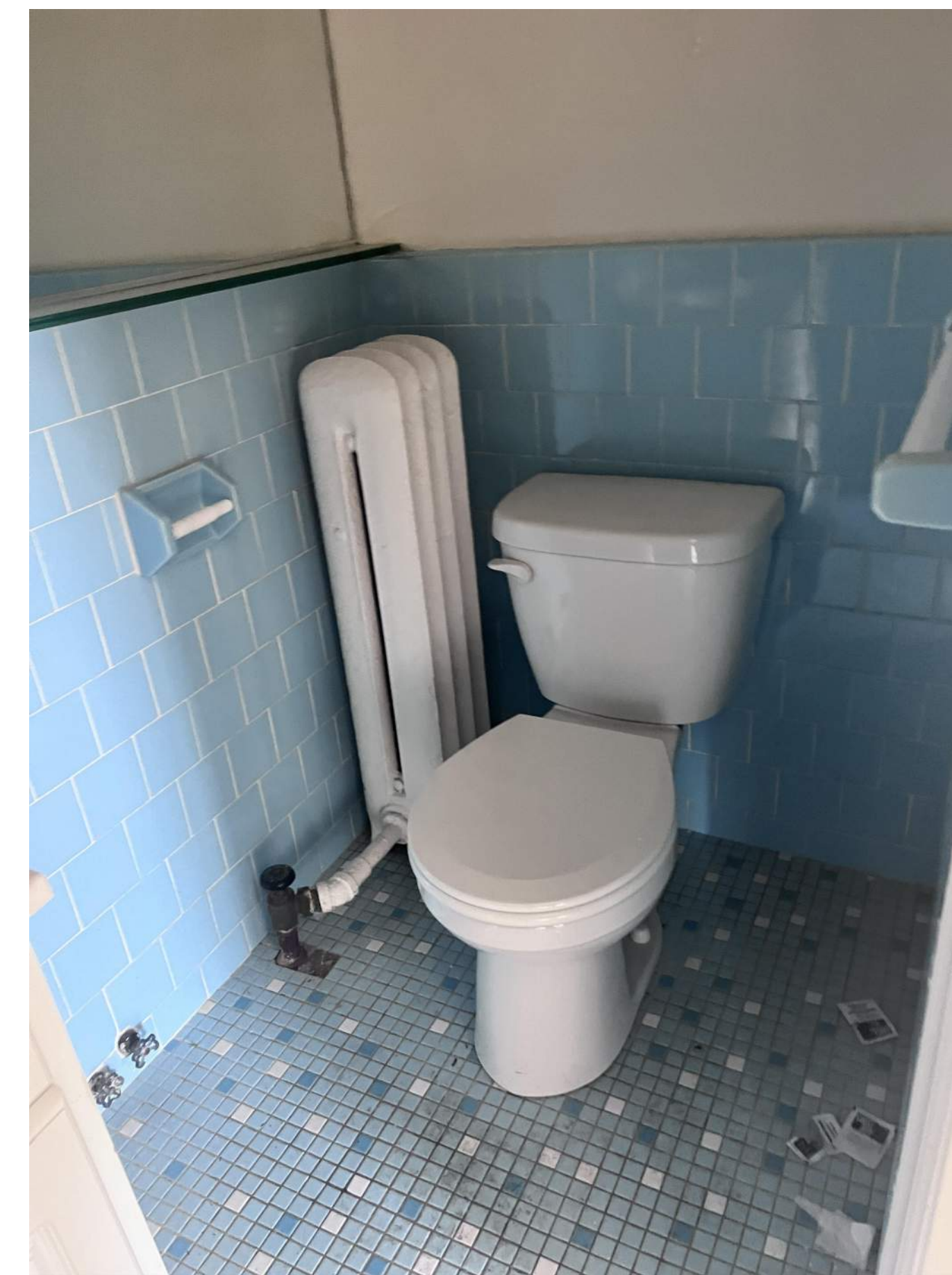
4. WATERSENSE LOW-FLOW FIXTURES THROUGHOUT
