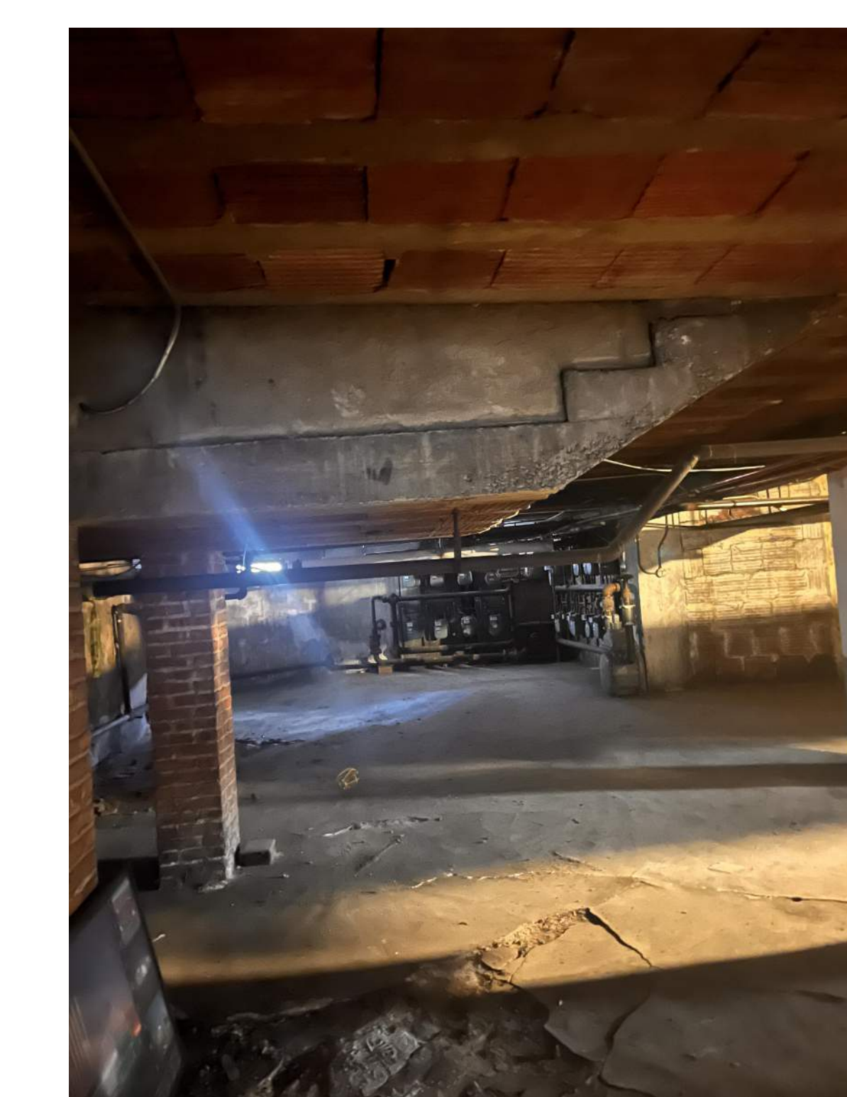
10. BASEMENT FLOOR DAMAGE
