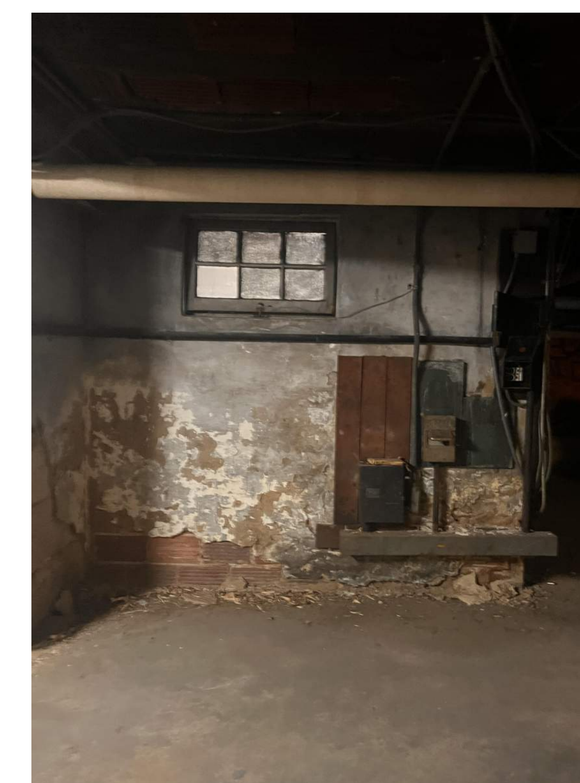
8. EQUIPMENT AND DAMAGED WALL AT BASEMENT
