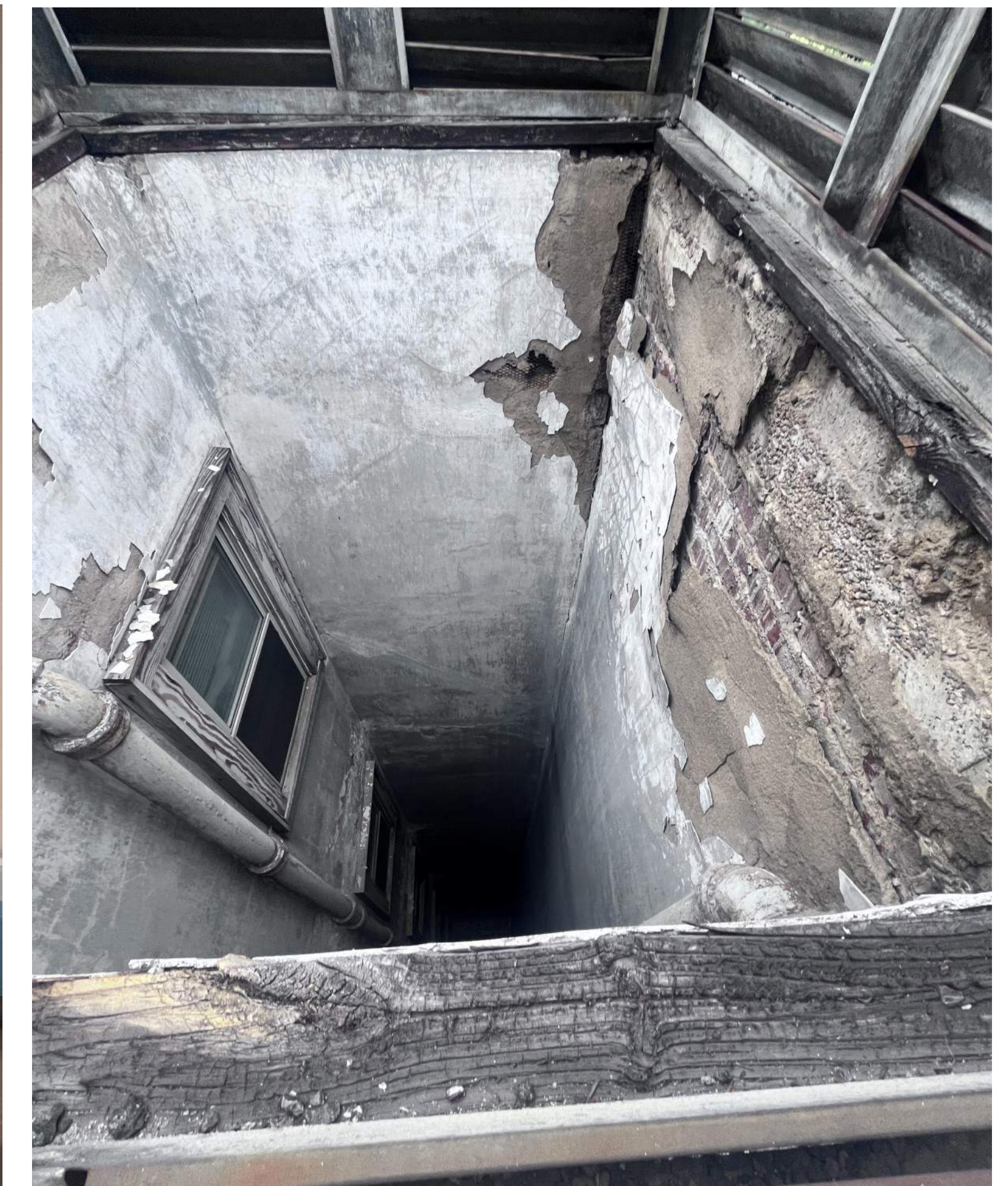
10. REPAIR VENTILATION SHAFT WALLS AND WATER INTRUSION ISSUE
