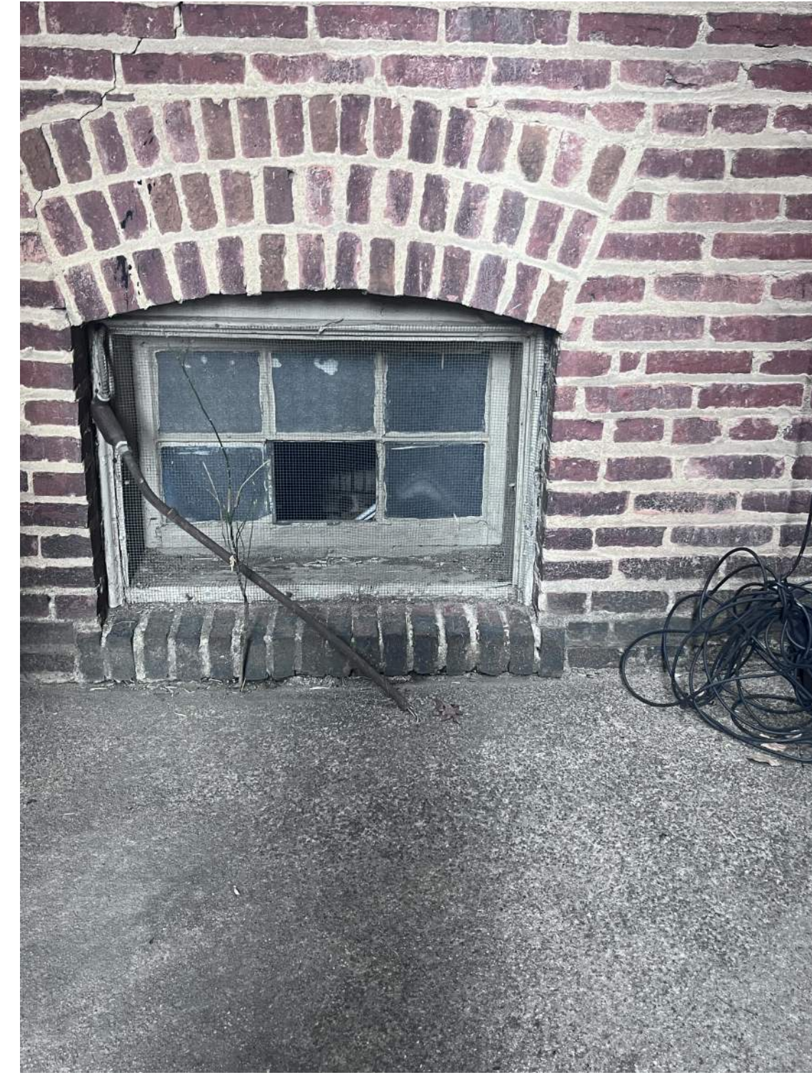
1. REPLACE BROKEN WINDOW AT BASEMENT
