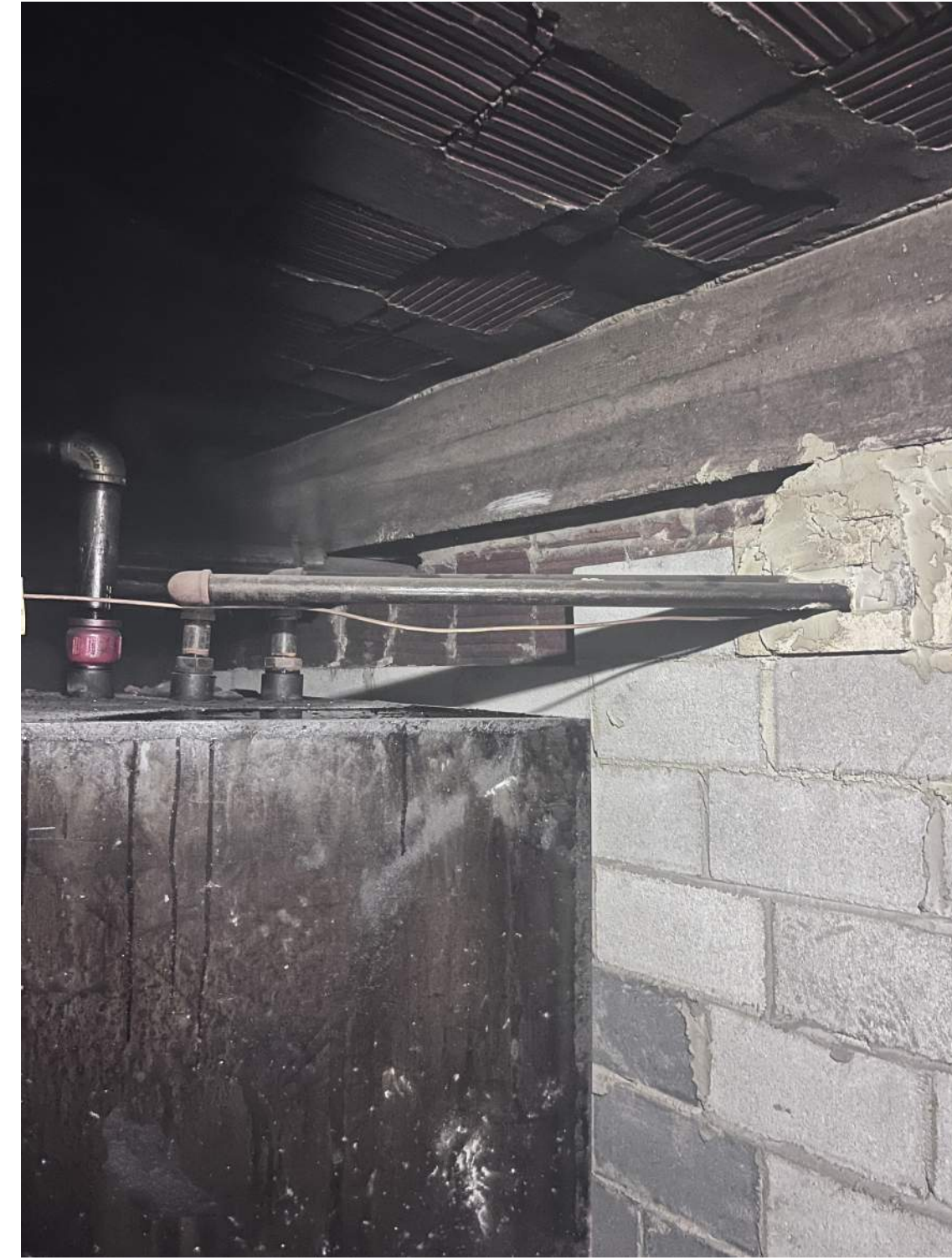
2. HAZARDOUS DIESEL TANK AT BASEMENT
