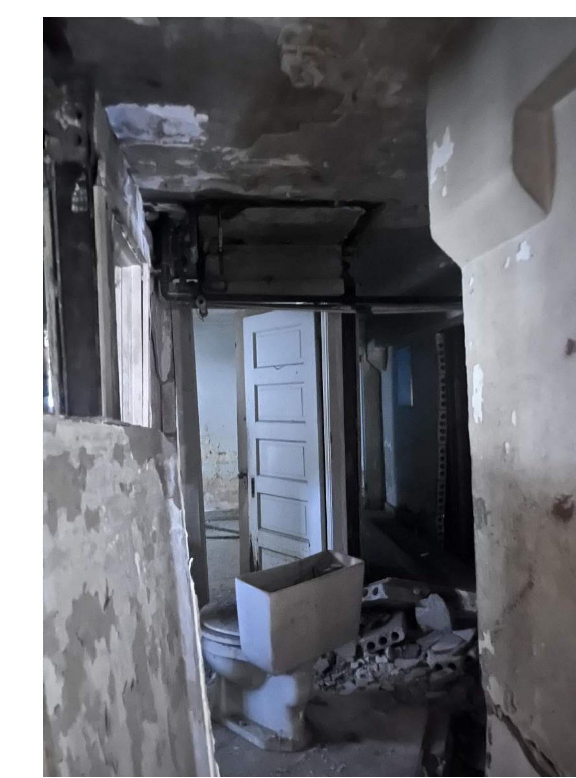
9. DAMAGED WALLS, FLOOR AND CEILING AT BASEMENT
