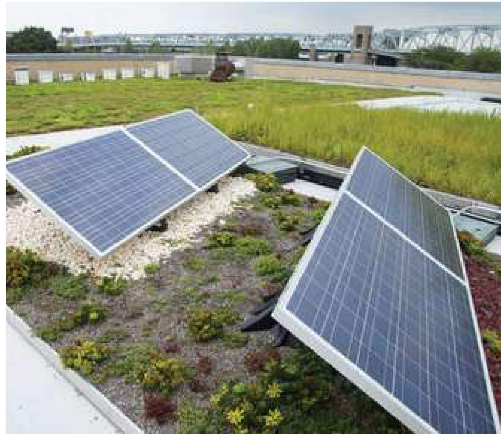
green roof and solar array
