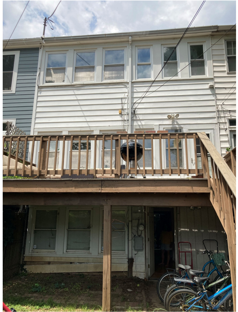
Board of Zoning Adjustment EXISTING REAR FACADE CITY OF CHICAGO CASE NO.20738 EXHIBIT NO.5
