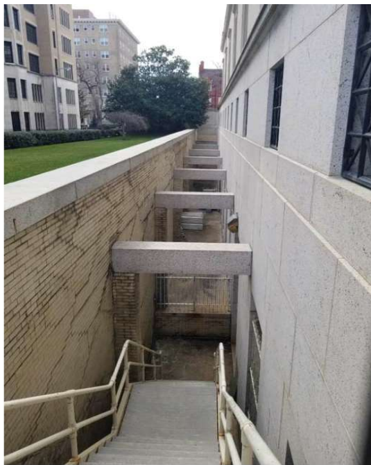
SCOTTISH RITE TEMPLE 1733 16TH STREET (HISTORIC DISTRICT) VIEW OF AREAWAY ON ALLEY
