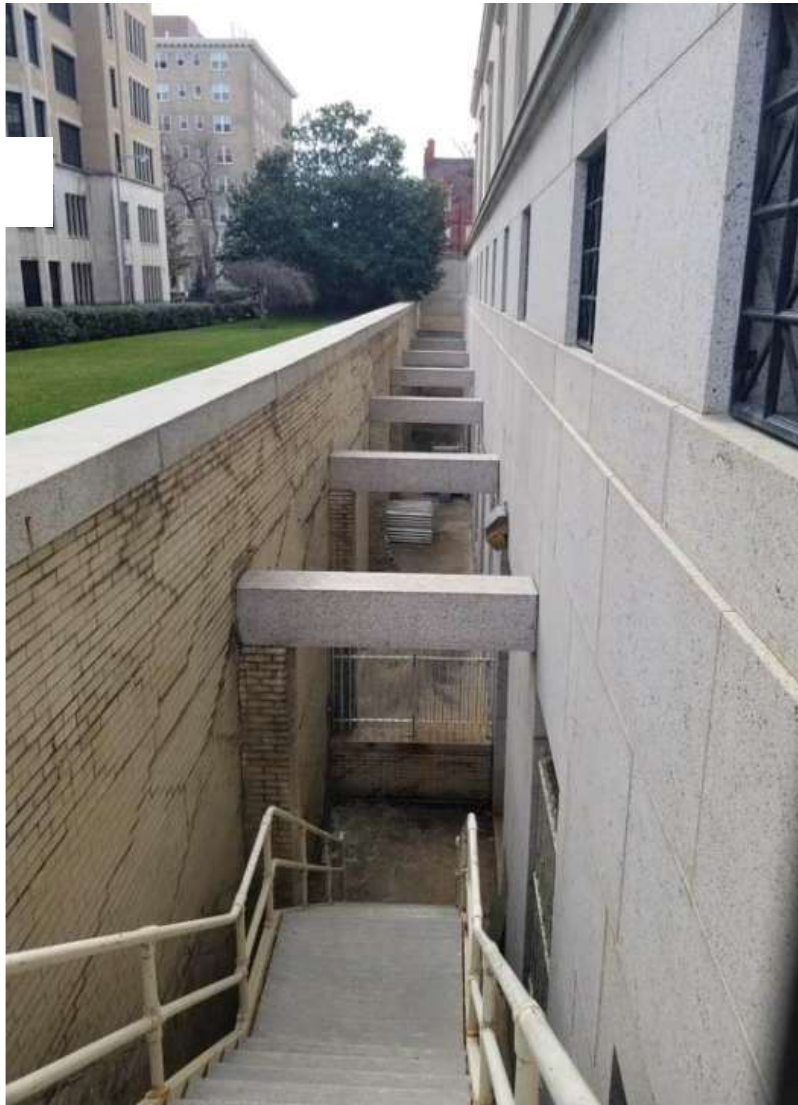
SCOTTISH RITE TEMPLE 1733 16TH STREET (HISTORIC DISTRICT) VIEW OF AREAWAY ON ALLEY
