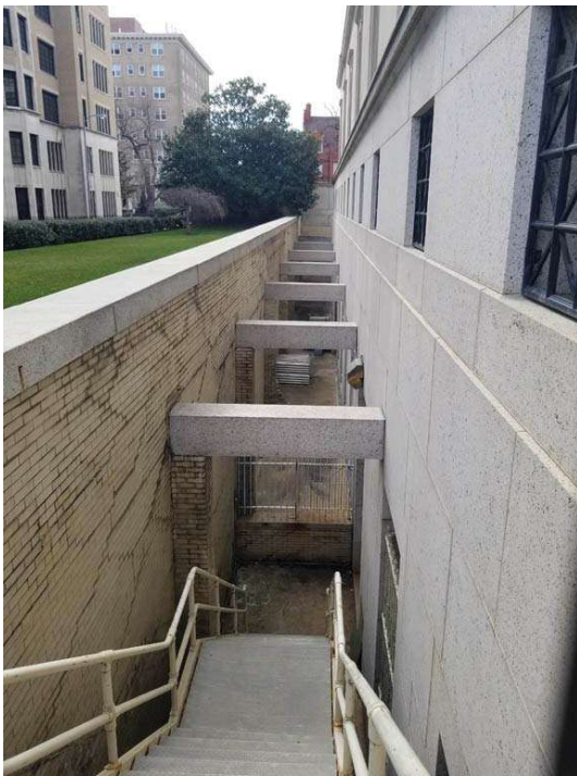
SCOTTISH RITE TEMPLE 1733 16TH STREET (HISTORIC DISTRICT) - VIEW OF AREAWAY ON ALLEY
