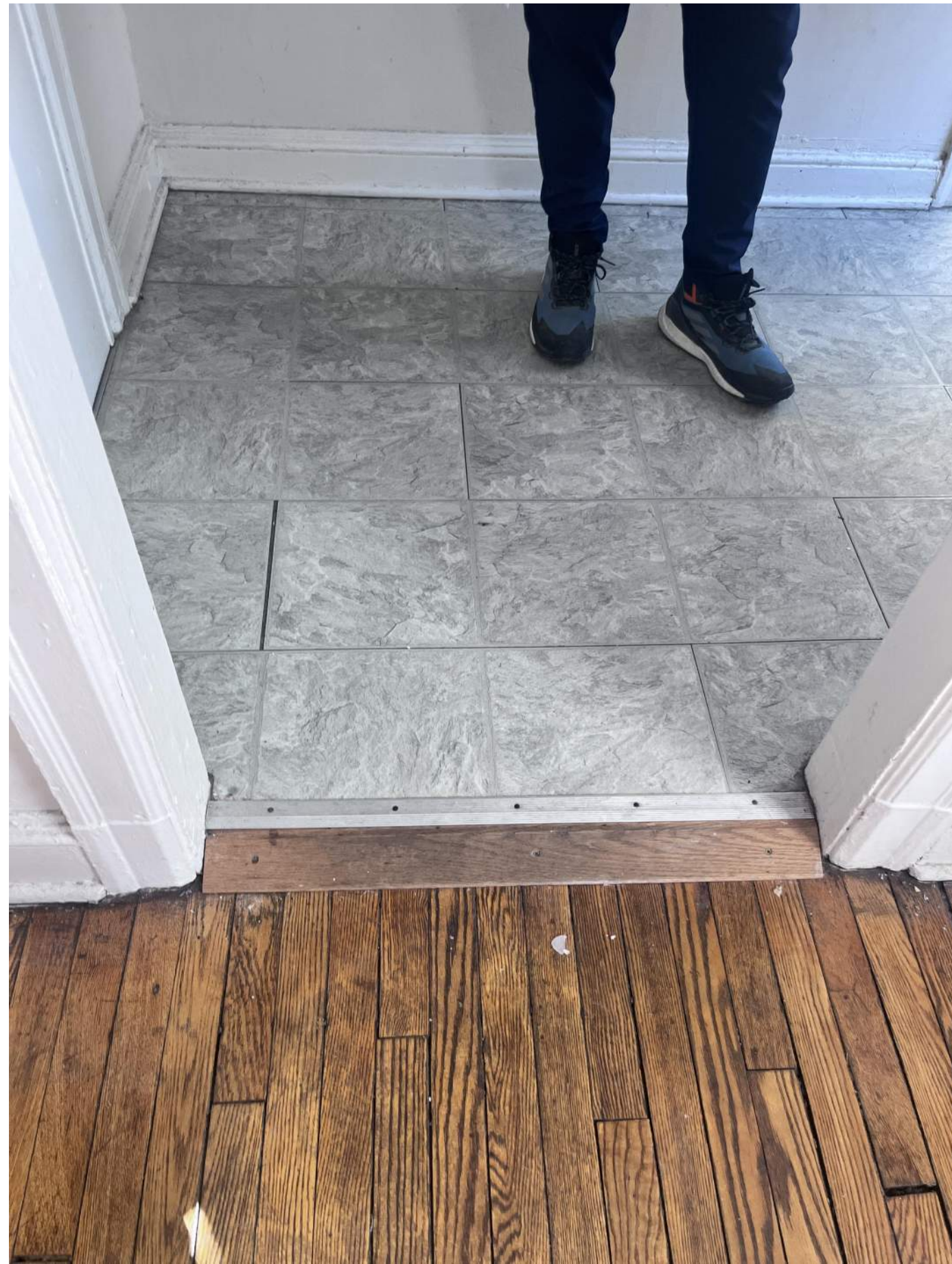
3. REPAIR & REPLACE DAMAGED FINISHES THROUGHOUT
