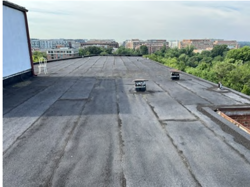
Deteriorating roof system – proposed complete roof replacement to address current water intrusion into 5 th floor
