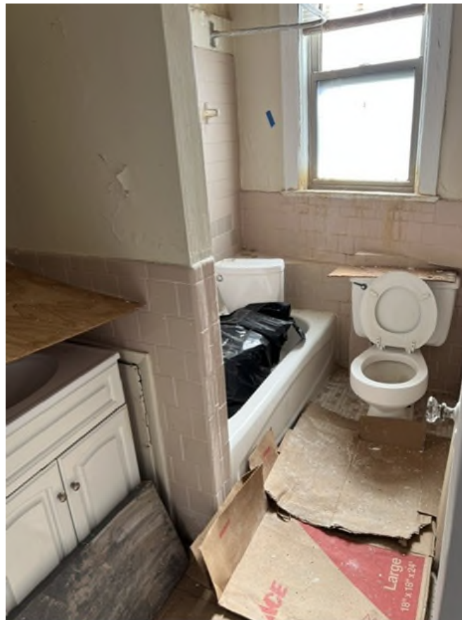
Interior water damage in unit
