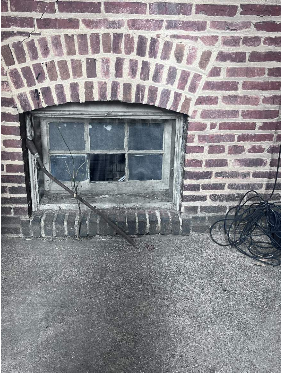
1. REPLACE BROKEN WINDOW AT BASEMENT
