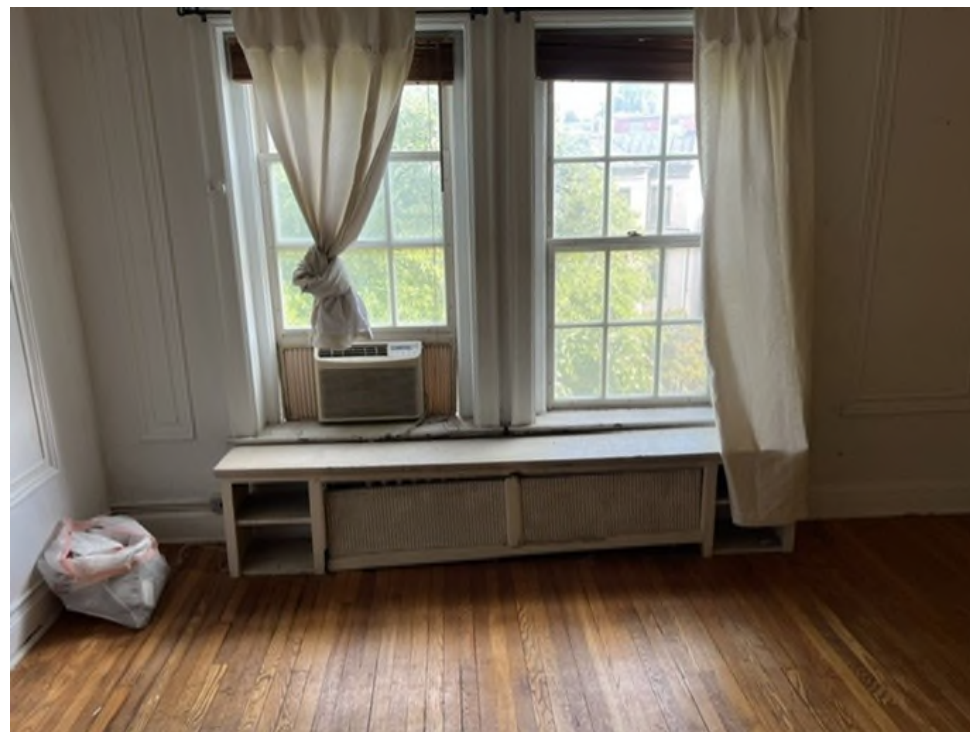
Dilapidated unit conditions with window unit AC and furnace radiator heat – proposed full replacement with modern, energy efficient HVAC system
