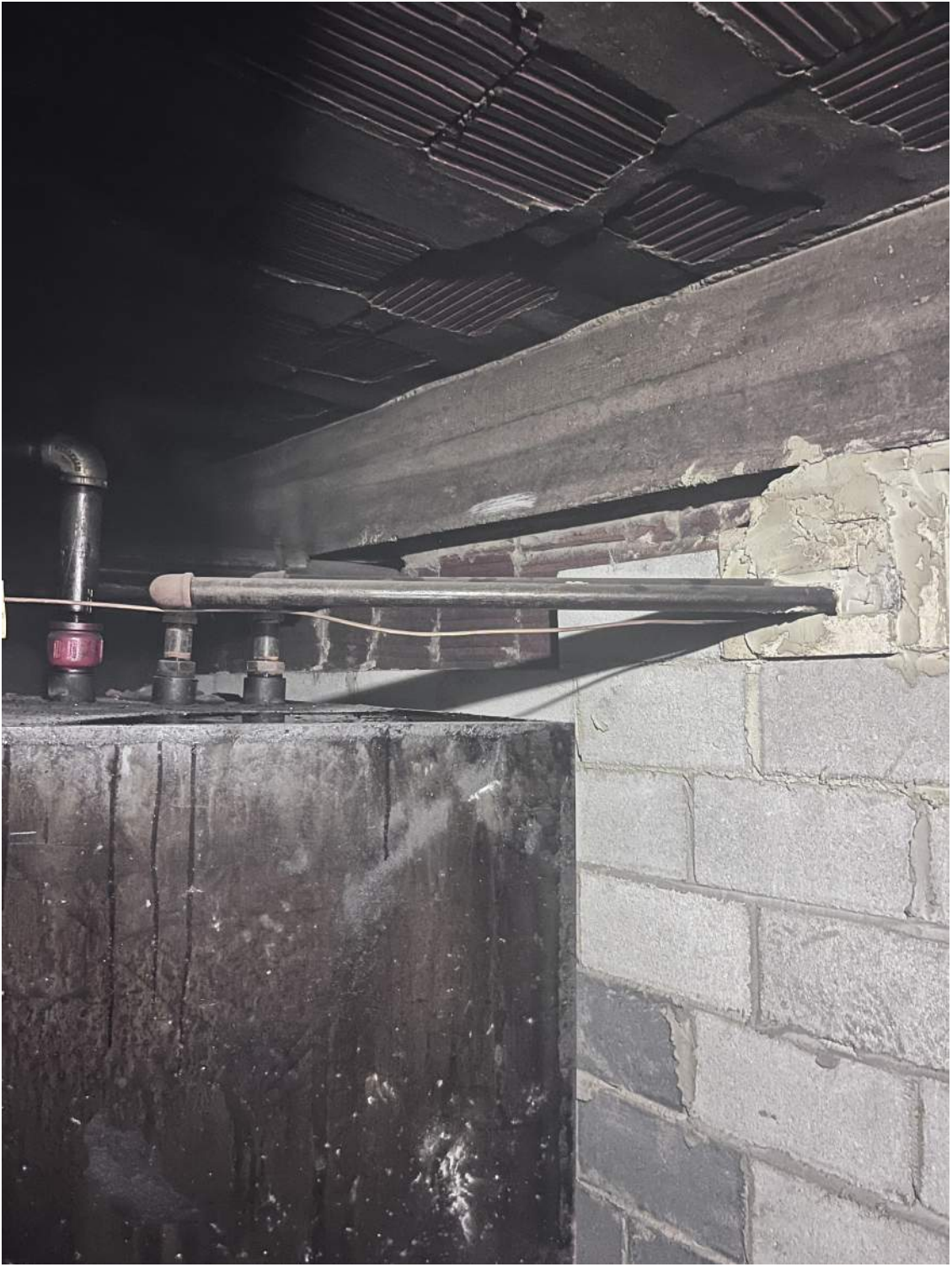
2. HAZARDOUS DIESEL TANK AT BASEMENT
