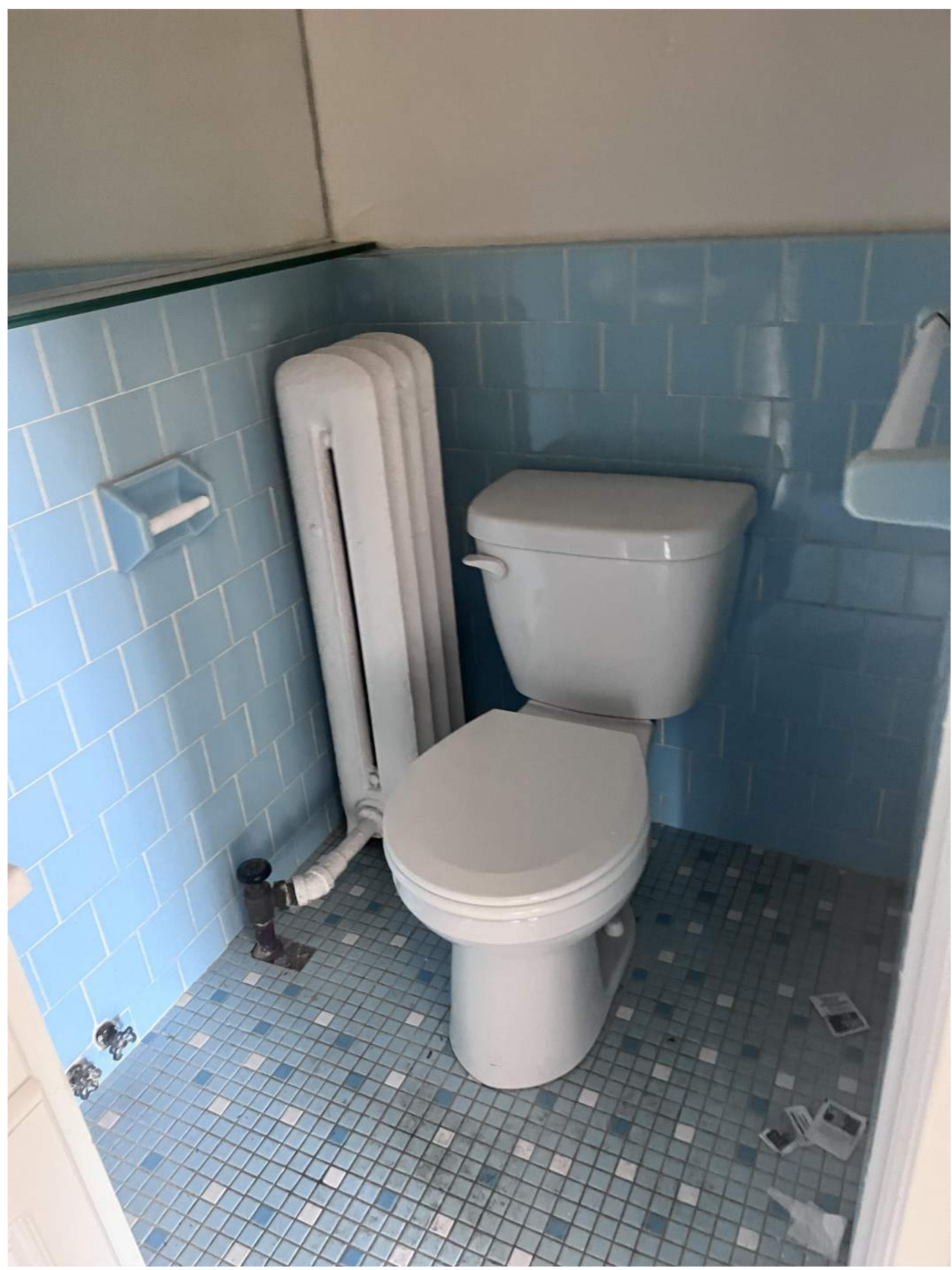
4. WATERSENSE LOW-FLOW FIXTURES THROUGHOUT
