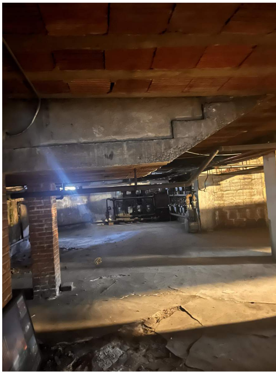
10. BASEMENT FLOOR DAMAGE
