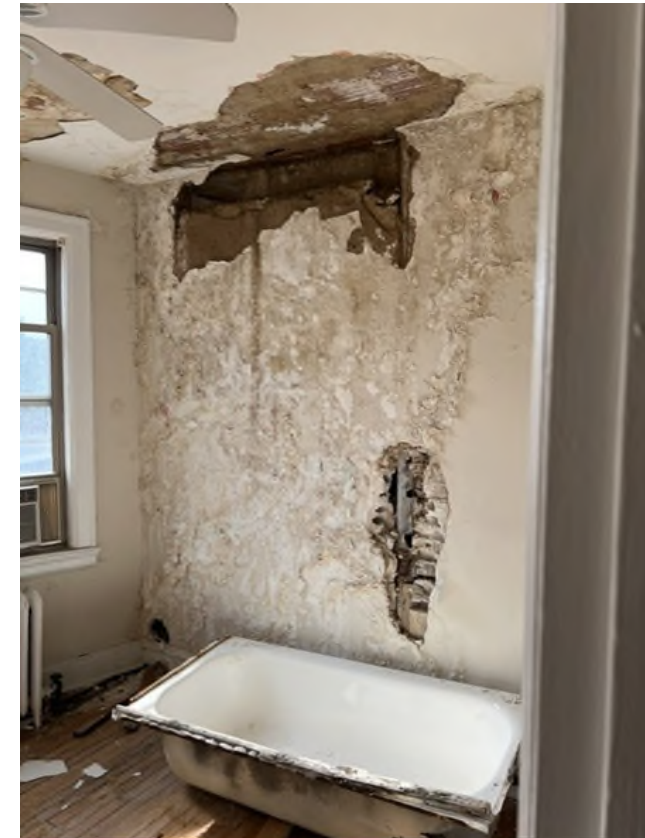
Interior water damage in unit
