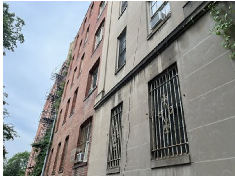
Poorly maintained historic façade with exposed and unsecure cable wires
