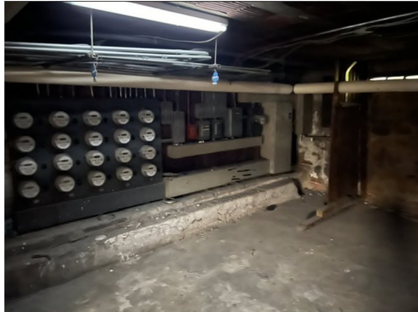
Dated and undersized electric/metering system – proposed full update and replacement with new, efficient and sustainable green electrical system
