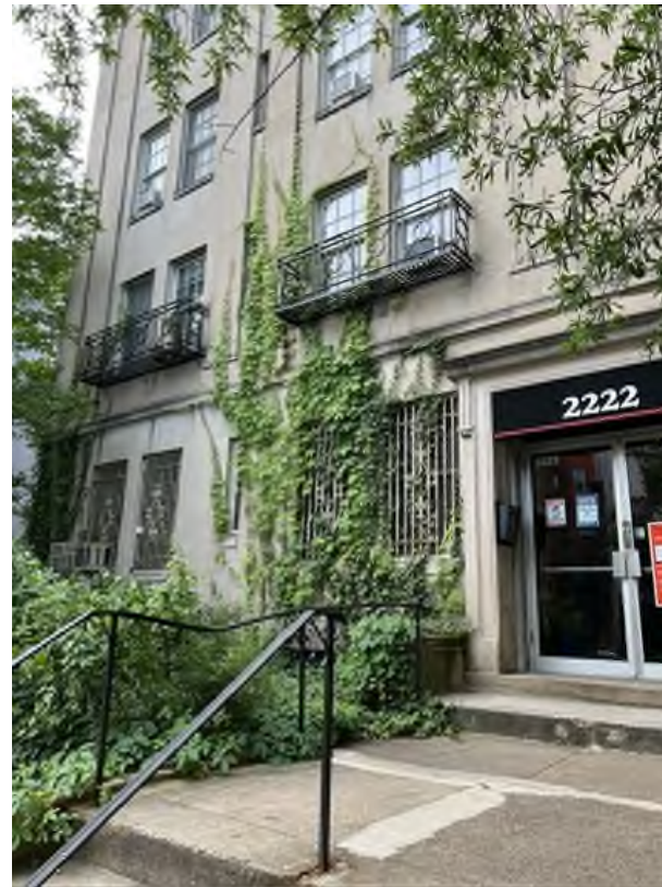
Poorly maintained historic façade with significant overgrowth
