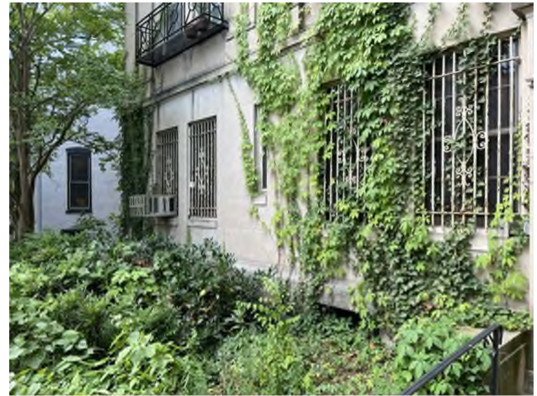
Poorly maintained historic façade with significant overgrowth
