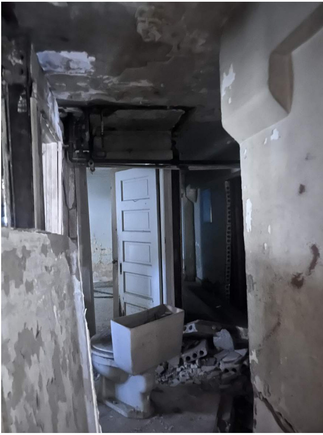
9. DAMAGED WALLS, FLOOR AND CEILING AT BASEMENT
