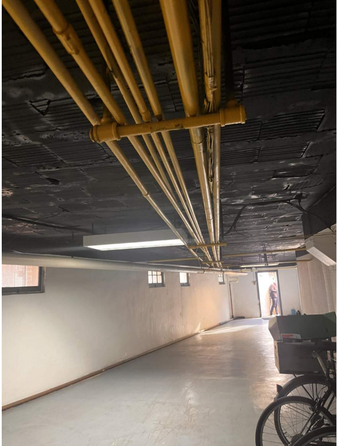
6. LOW CEILING HEIGHT AT BASEMENT
