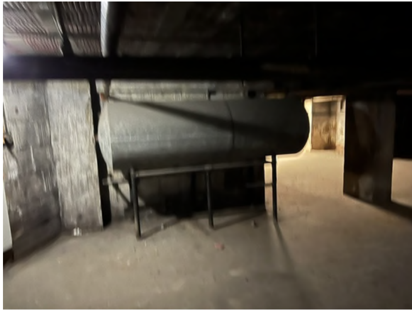
Above ground storage tank located in basement – proposed to be removed per Phase 1 Environmental Site Assessment Report
