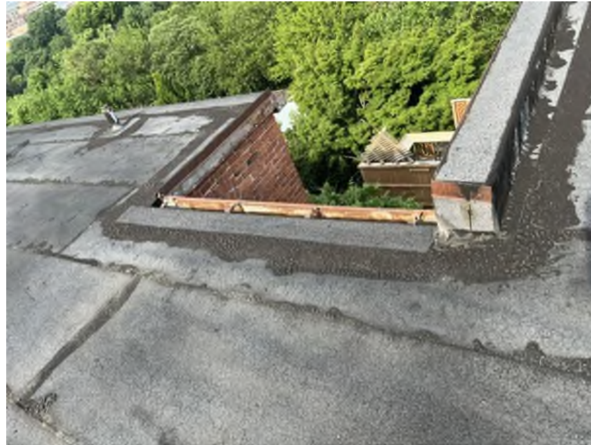
Severely rusted gutters – proposed to be replaced
