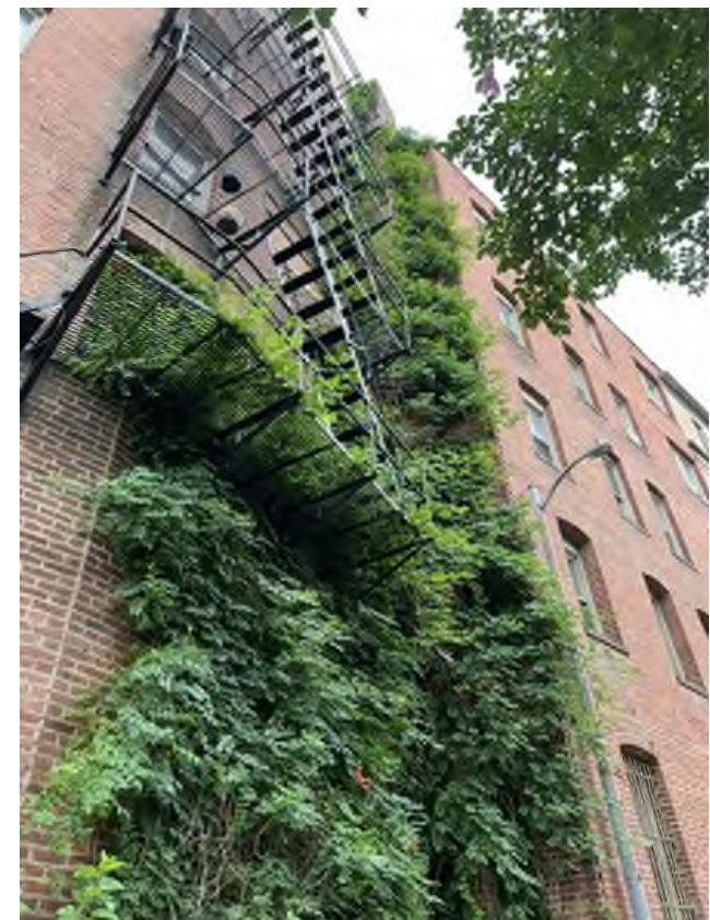
Poorly maintained and neglected exterior façade with significant overgrowth
