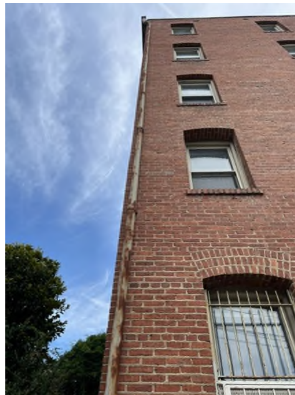
Severely rusted downspouts
