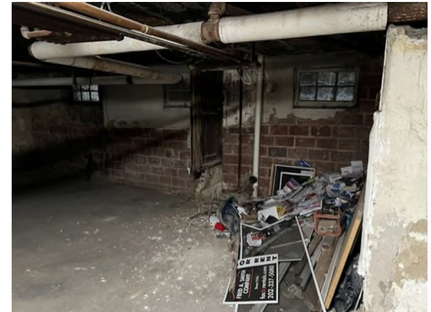
Deteriorated cellar condition
