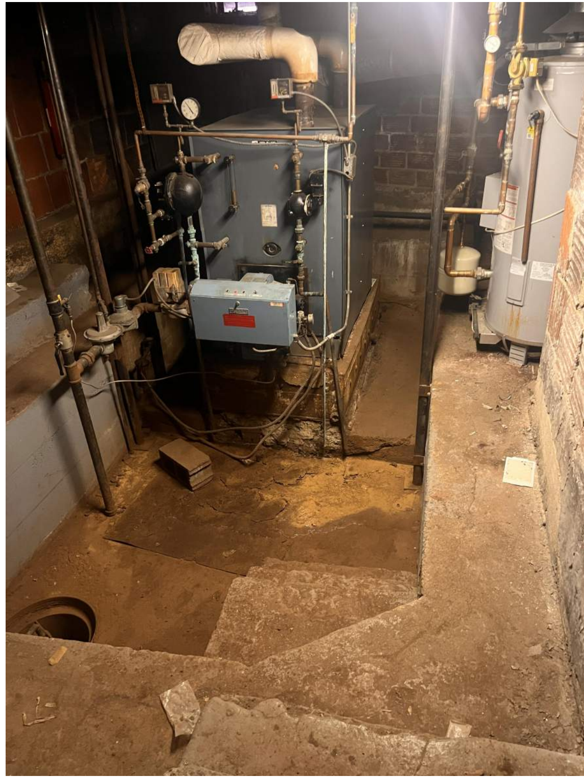
7. UTILITY ROOM AT BASEMENT
