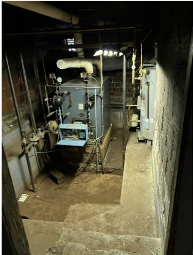
Dated gas furnace heating system – proposed replacement with modern, energy efficient HVAC system
