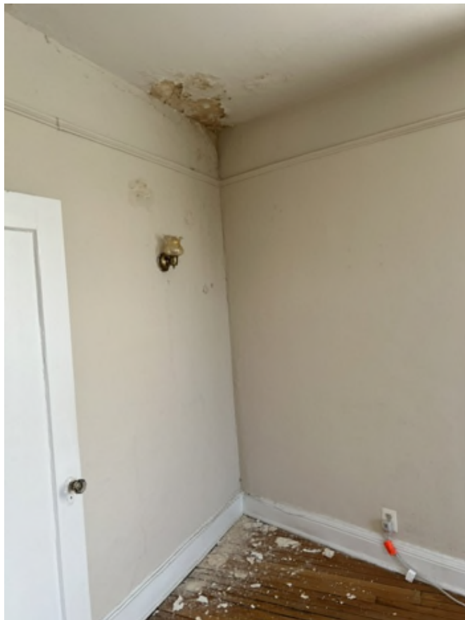
Interior water damage in unit
