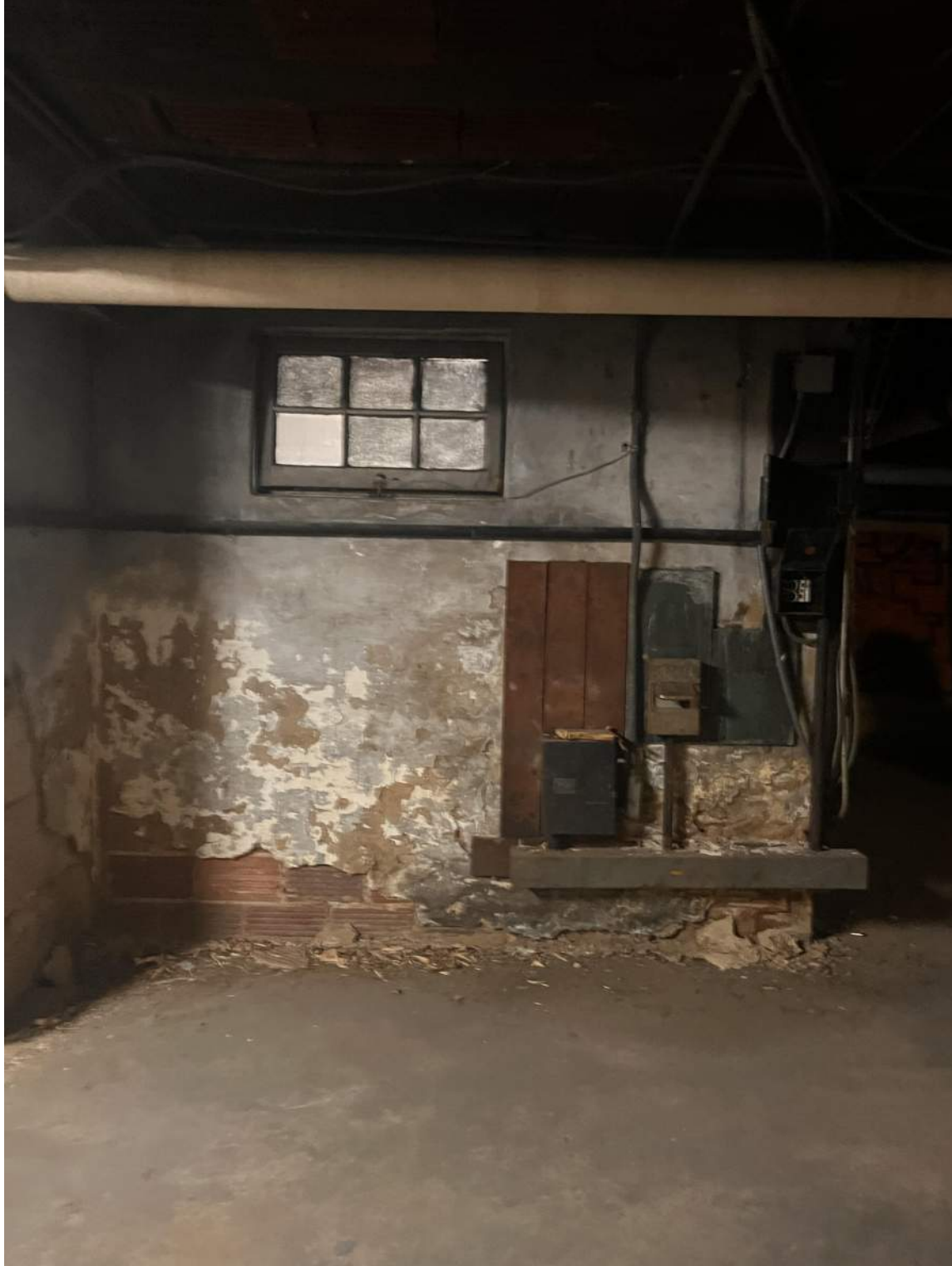
8. EQUIPMENT AND DAMAGED WALL AT BASEMENT
