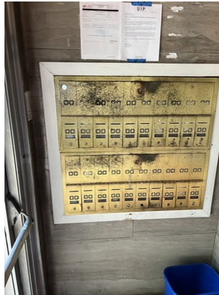
Rusting resident mailbox
