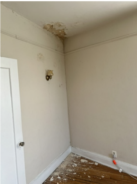
Interior water damage in unit
