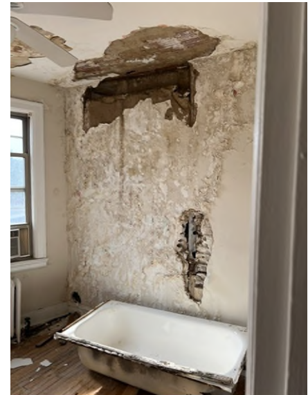
Interior water damage in unit
