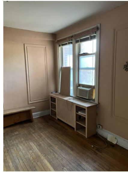
Dated interiors with window unit AC and furnace radiator heat – proposed full replacement with modern, energy efficient HVAC system
