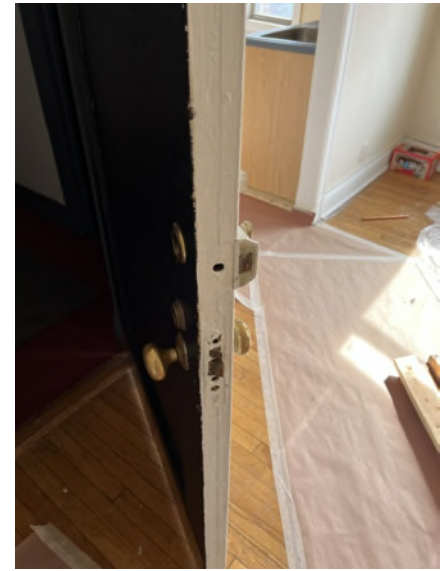
Dated unit doors and security features
