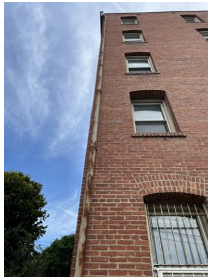
Severely rusted downspouts
