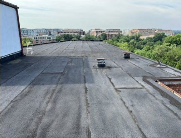
Deteriorating roof system – proposed complete roof replacement to address current water intrusion into 5 th floor
