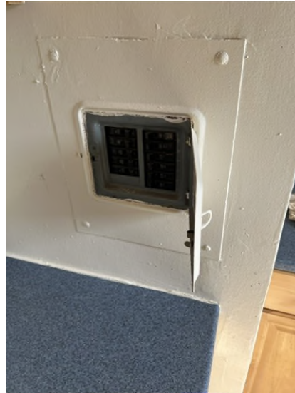
Dated and undersized electrical breaker panel – proposed full replacement with new, efficient and sustainable green electrical system
