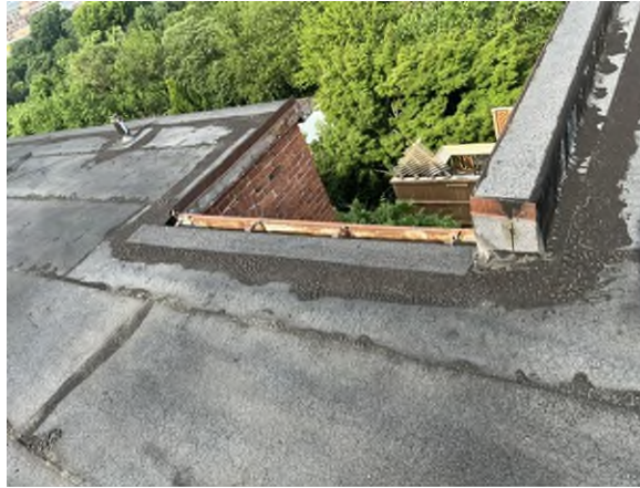
Severely rusted gutters – proposed to be replaced
