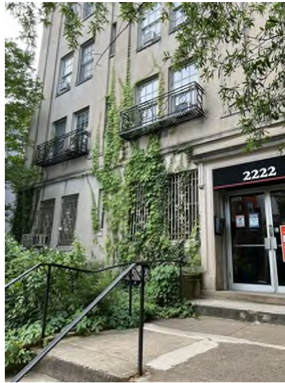
Poorly maintained historic façade with significant overgrowth
