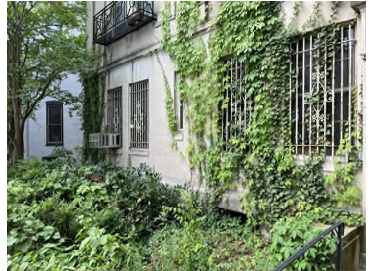
Poorly maintained historic façade with significant overgrowth
