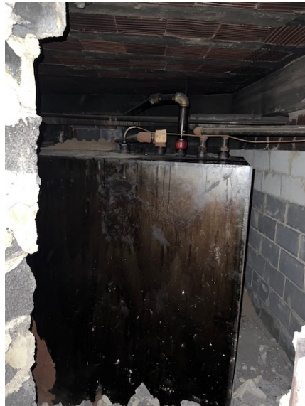
Above ground storage tank located in basement – proposed to be removed per Phase 1 Environmental Site Assessment Report
