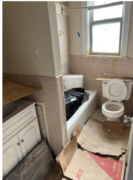
Interior water damage in unit
