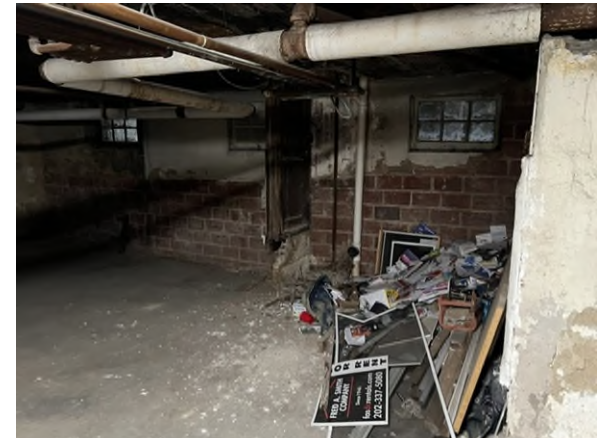
Deteriorated cellar condition
