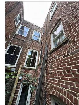
VIEW OF DOGLEG CONDITION FROM GROUND LEVEL
