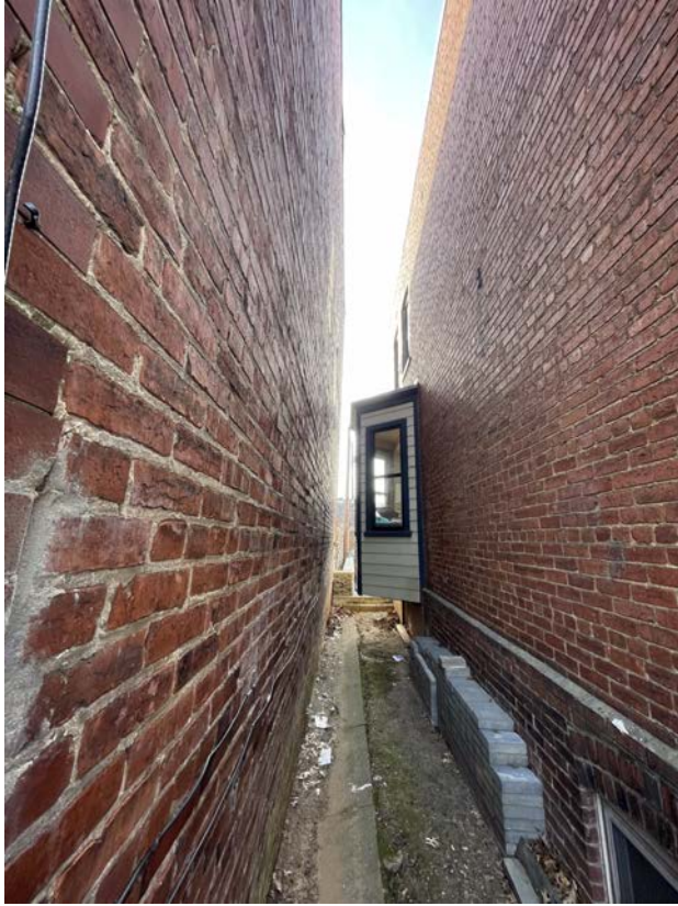
The narrow side walkway between the western wall of the 932 Shepherd Street (left) and 934 Shepherd Street (right), showing the close proximity of the two structures — 18 inches.
