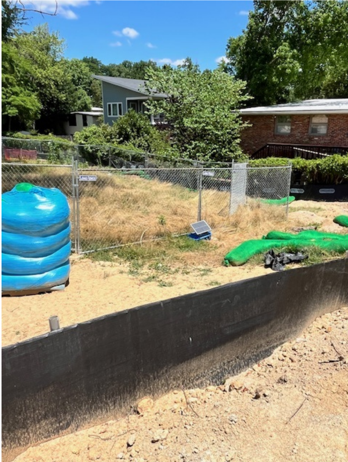
Figure 10: Vibration Monitoring – UM14249
