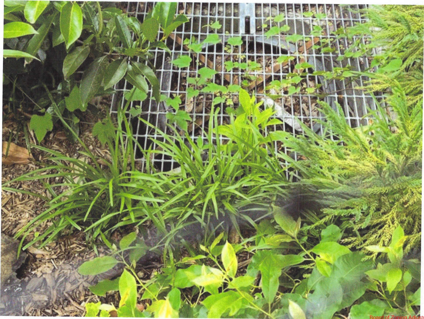
Storm drain covered with debris
