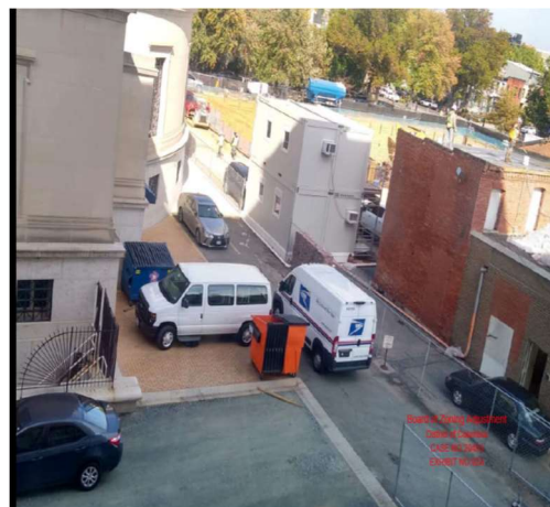
Photo taken by Wendy Schumacher showing the construction site, delivery area and new temporary parking area directly below her windows.
