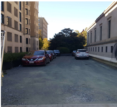
The new temporary parking lot built between the Chastleton and the Temple to accommodate vehicles during the construction. It is built almost under the bedroom windows of the residents of the Chastleton (shown on the left)
