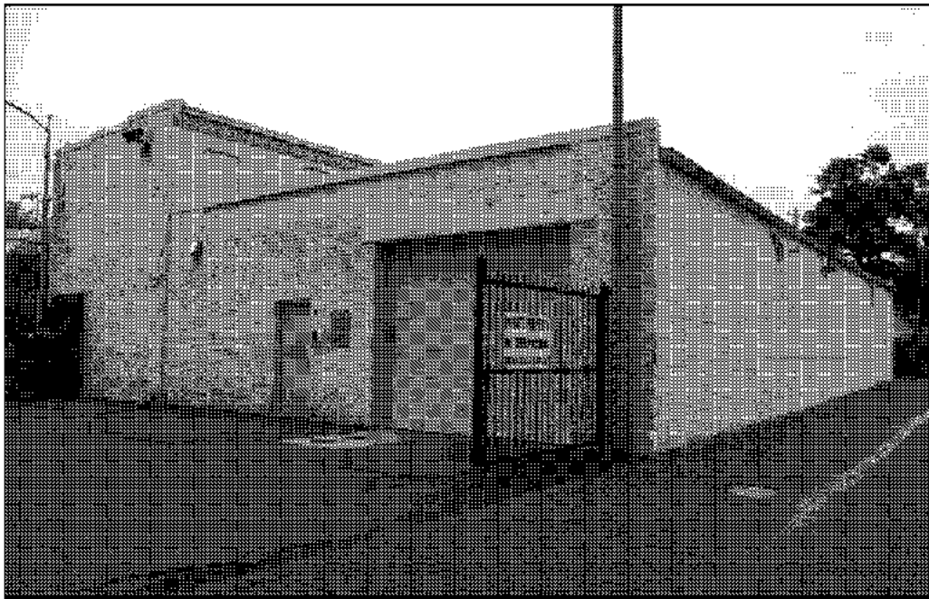
Figure 2: Scottish Rite Temple Garage, west and south elevations, facing northeast. EHT Tracerics.
