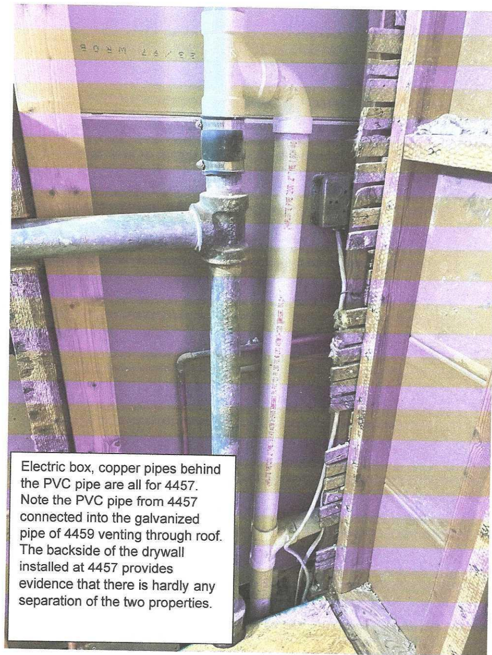
Figure 1 Electric, plumbing, vent inside the common wall 4457-4459
