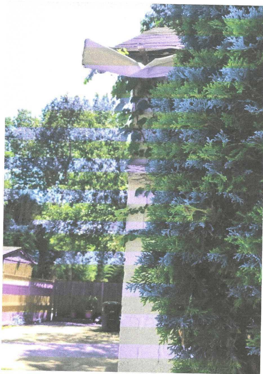
Damage to garage/gutter at 4459 from prior construction at 4457
