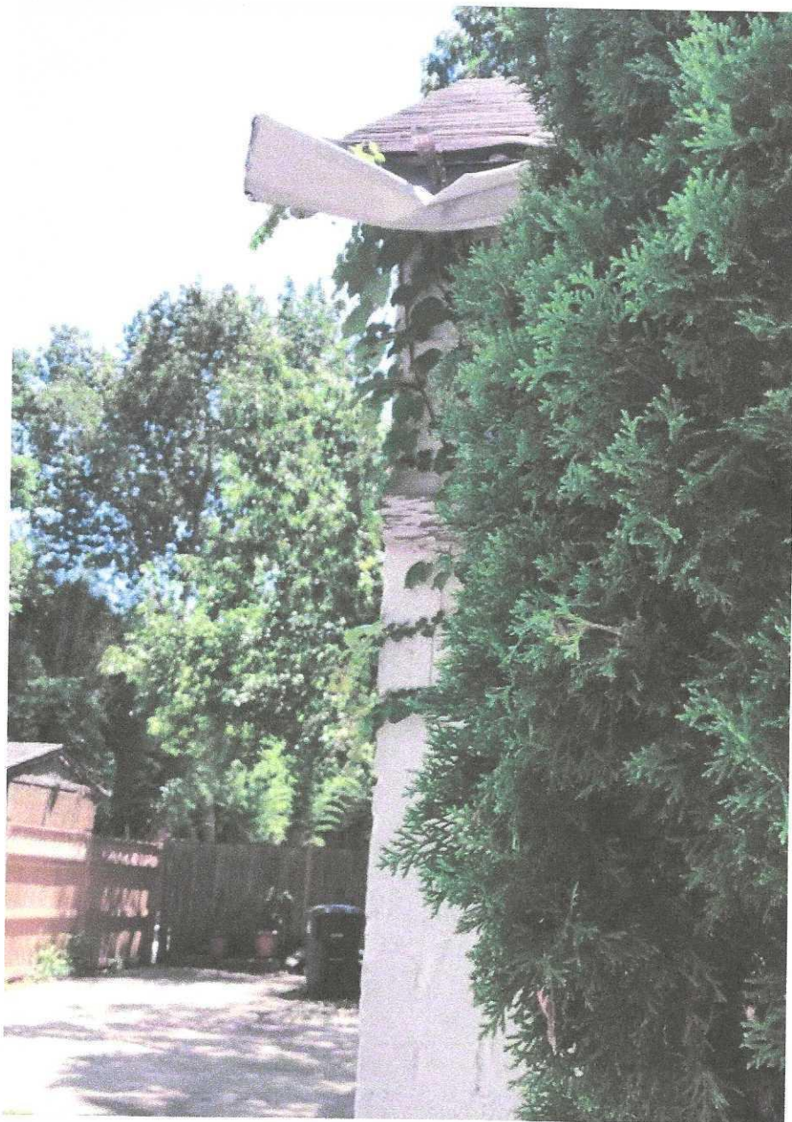
Figure 7 Damage to garage/gutter at 4459 from prior construction at 4457
