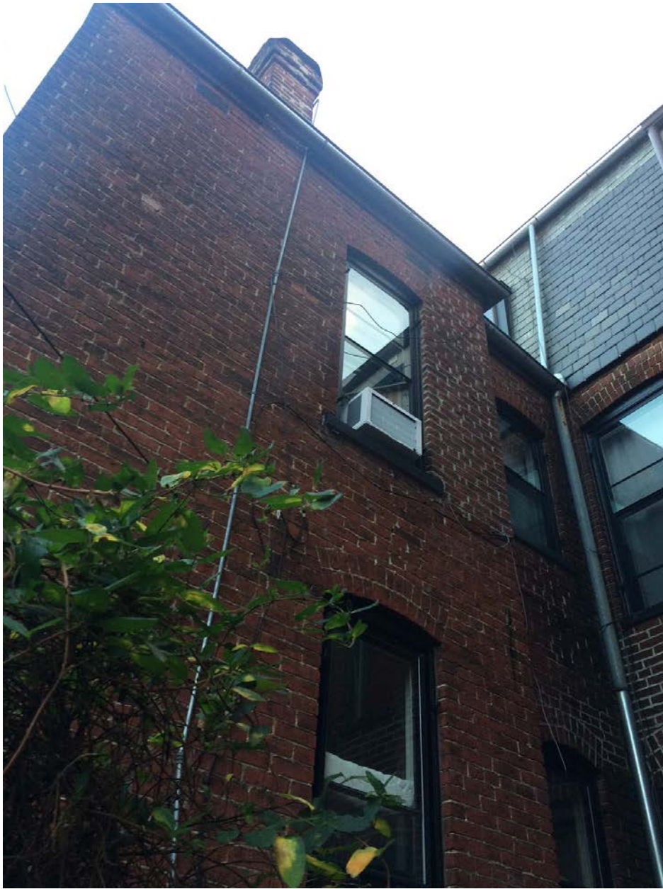
VIEW FROM OPEN COURT @ 1016 MASS AVE NE, LOOKING TOWARD 1018 MASS AVE NE
