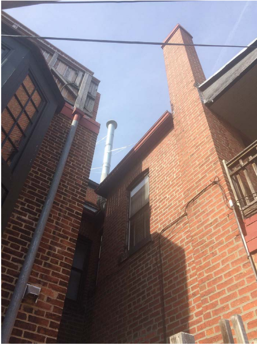
VIEW FROM REAR YARD @ 1016 MASS AVE NE, LOOKING TOWARD 1014 MASS AVE NE
