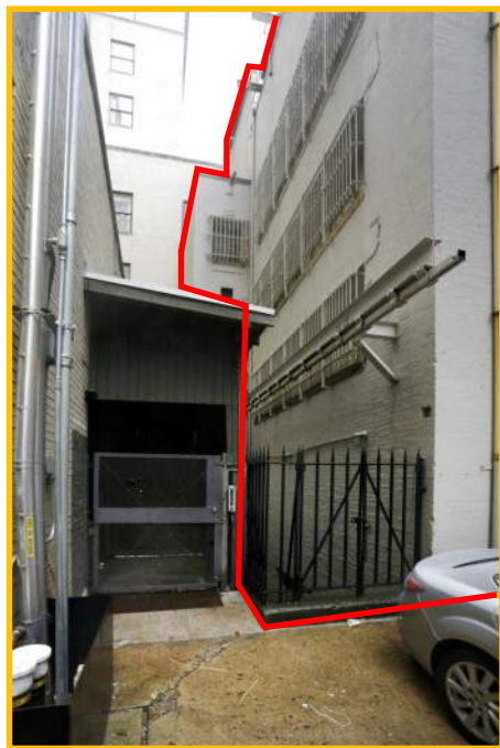
ENLARGED VIEW OF EXISTING NON-COMPLIANT REAR YARD
