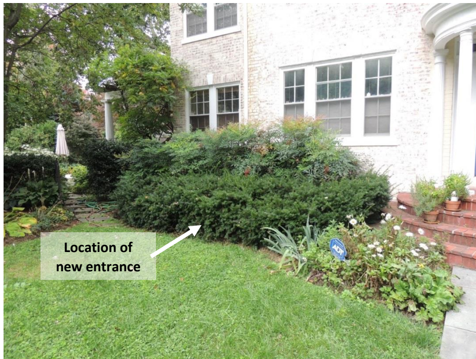
View of the south elevation, at the location of the proposed entrance
