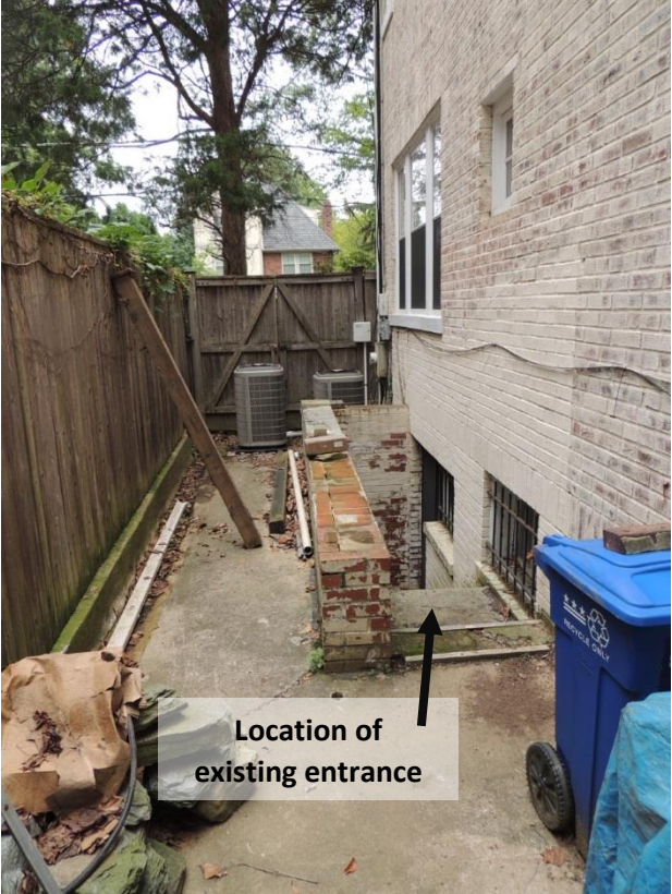
View of the Rear (North) Wall showing existing entrance to the basement
