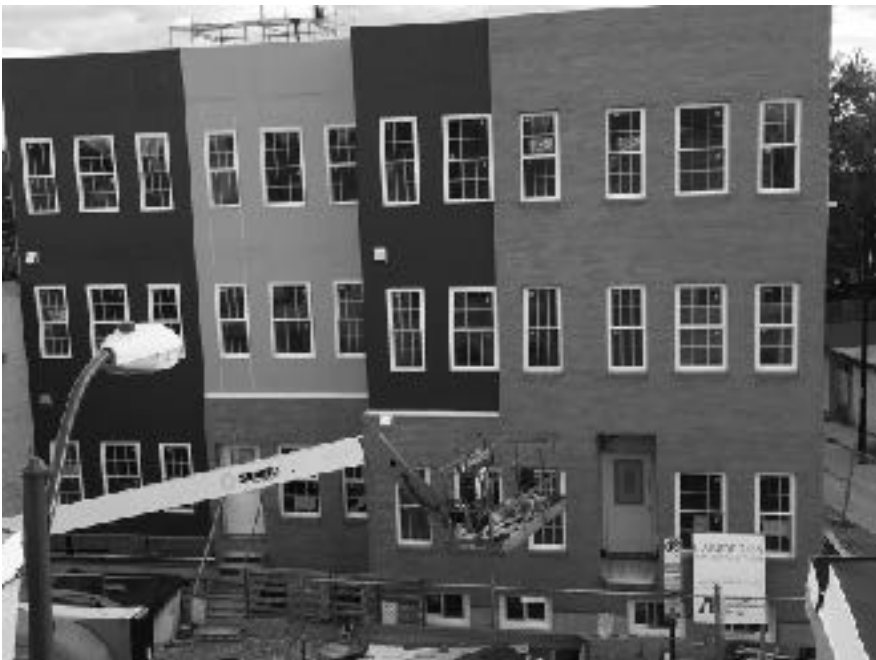
October 22, 2016: Structures spanning 410 and 412 Richardson Place NW. Permit board not erected.
