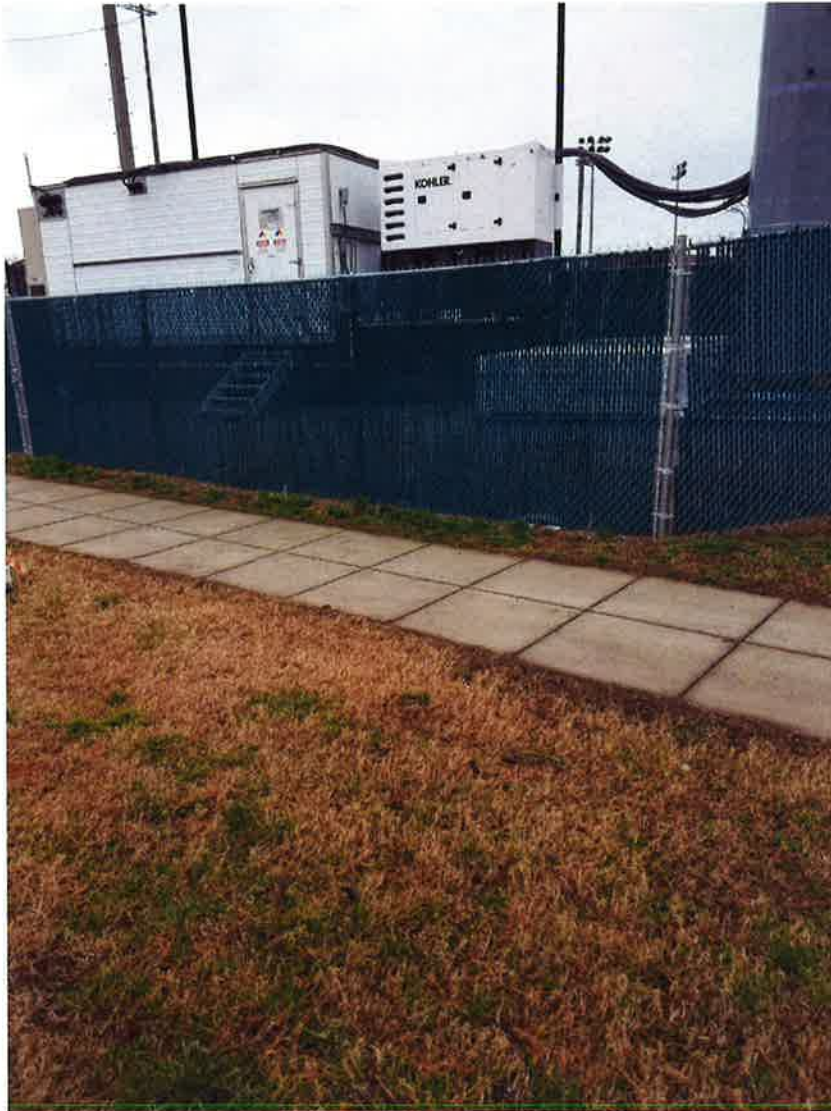
Picture 11 – Graffiti painted over – 2/26/18
