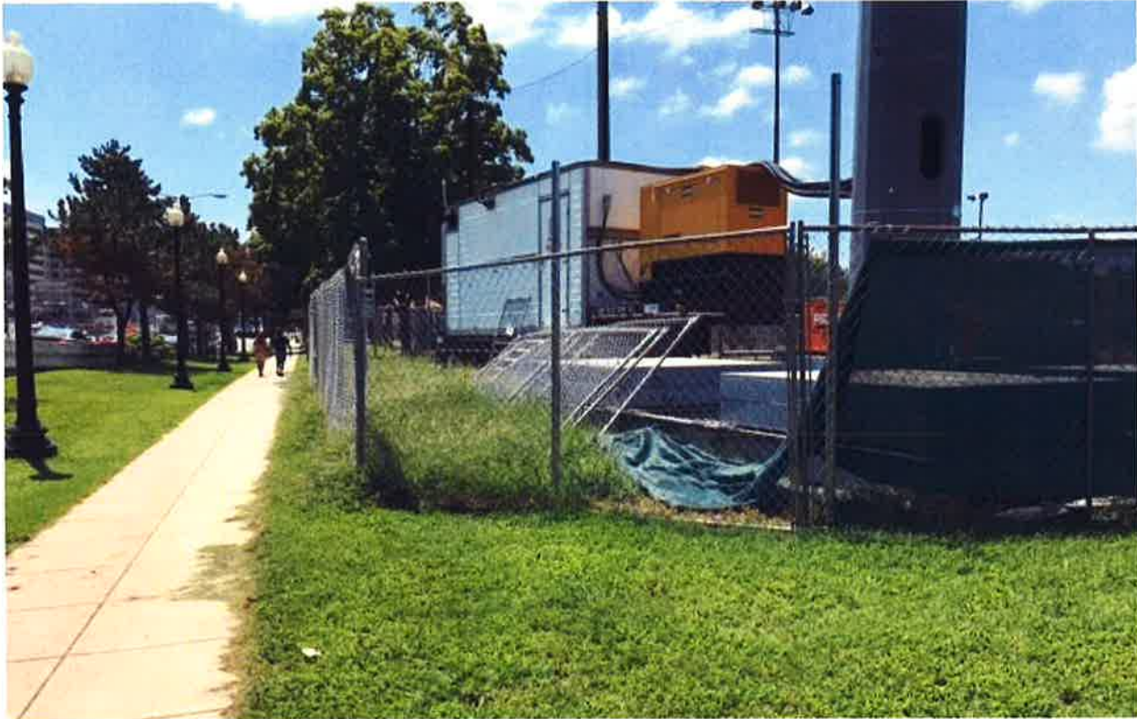
Picture 9 – Showing compound overgrowth in July 2017.
