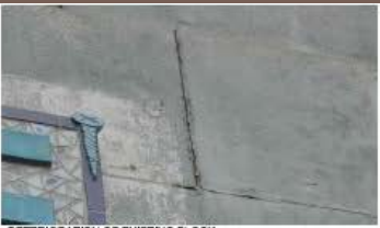
- DETERIORATION OF EXISTING BLOCK
