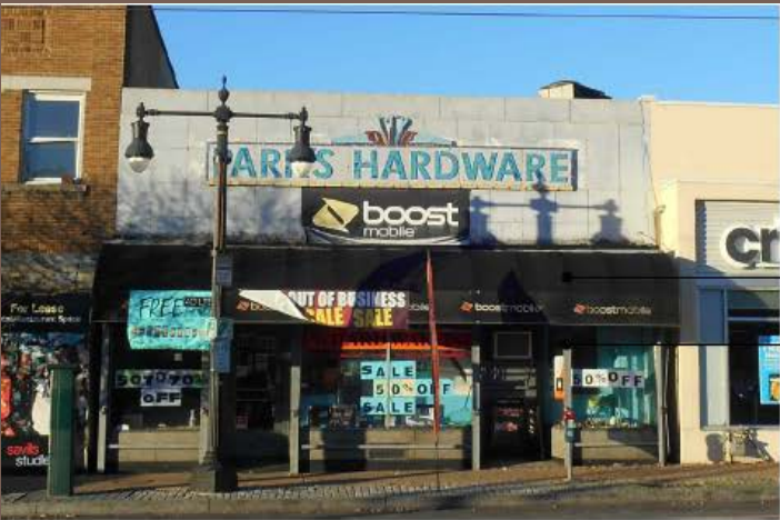
3 EXISTING FACADE CONDITION SCALE: 1/8" = 1'
