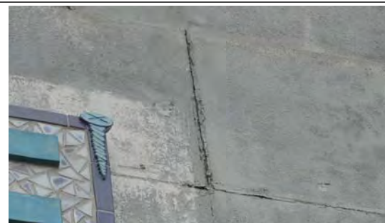
- DETERIORATION OF EXISTING BLOCK
