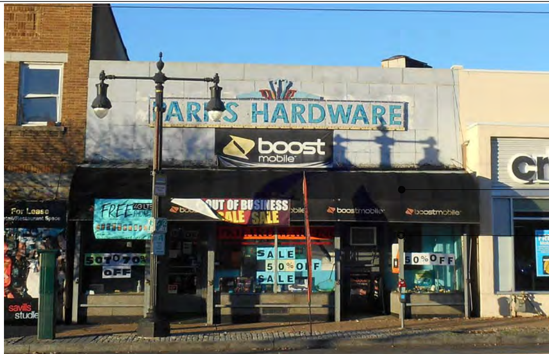
3 EXISTING FACADE CONDITION SCALE: 1/8" = 1'
