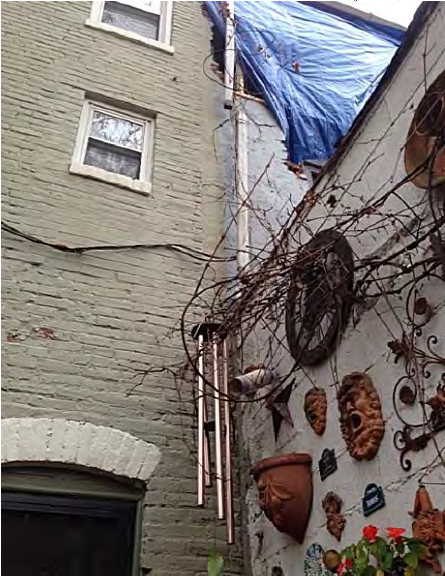
Attachment G - photo showing dangling downspout in imminent threat of falling at 518 6th St., NE
