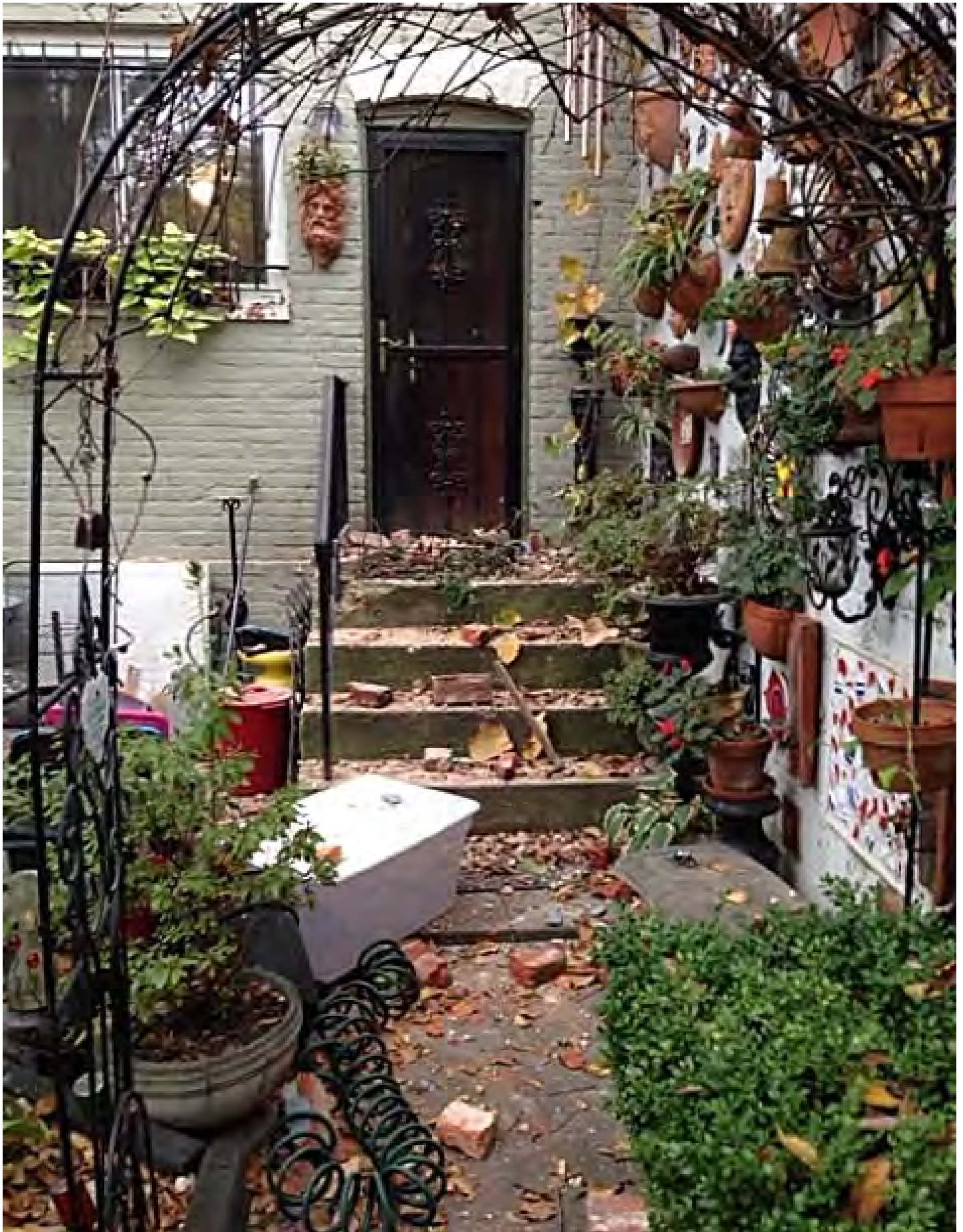
Attachment F - photo showing failure to protect adjoining property (520 6th St. NE) from falling bricks during demolition at 518 6th St., NE
