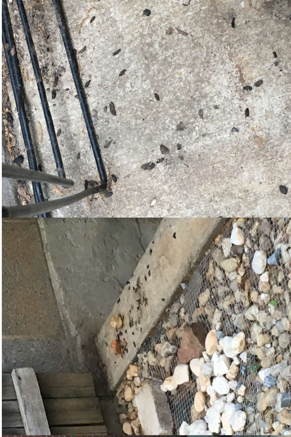
Feces, Food Waste, Abandoned Equipment Around Shed 2018
