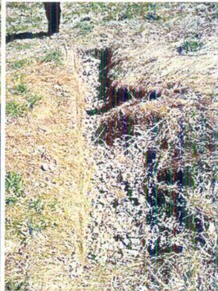
Septic tank effluent pipe and trough
