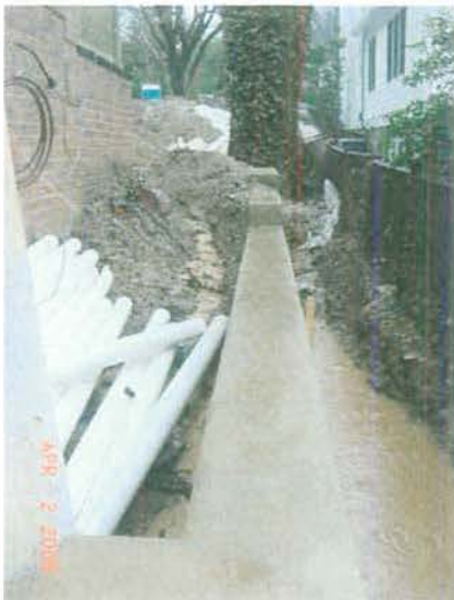
5524 MacArthur's silty runoff flows downhill to alley
