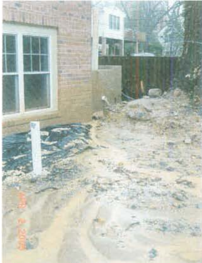
Pipe thru wall discharges to rear of 5524 MacArthur
