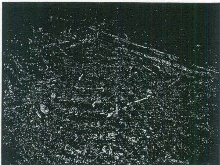
Silt puddle early fall 2004, during one of the many silt fence breaks.
