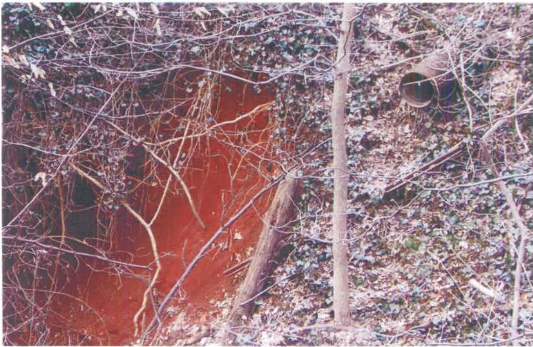
DRAINAGE Pipe from street to stream
