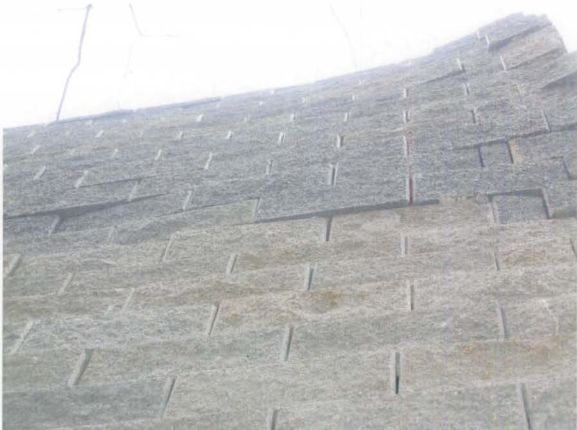
Illustration No. 3 (example of bulges, warps, and defects in exterior wall, Dec. 2004)
